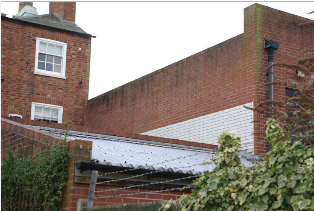
Plate 3. Party wall boundary between 50-56 and 58-60 New Walk, showing glazed brick wall, with rebuilt parapet above tied into Wellington Street façade. Looking west.
