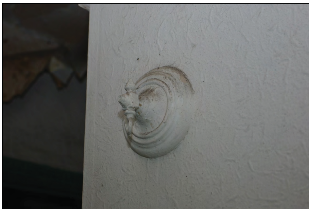
Plate 23. Early gas light fitting on attic level landing. Looking east.
