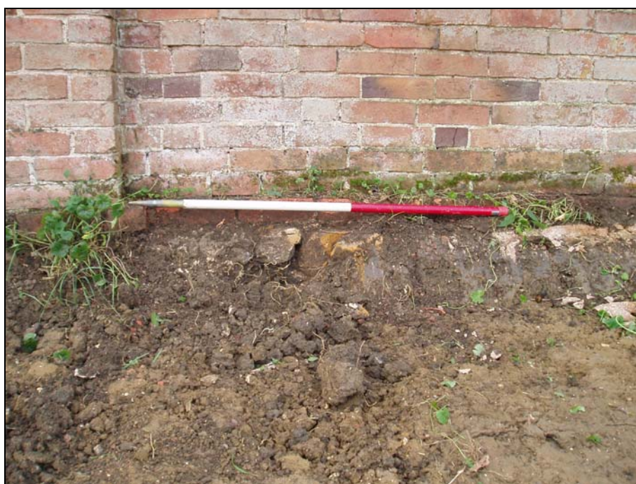
Plate 28. Ironstone block footings to garden wall, revealed by topsoil stripping. Looking west.
