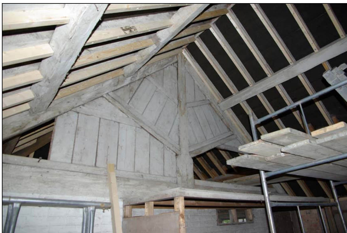
Plate 14. Remains of closed truss between sleeping quarters and first floor storage. Looking west.
