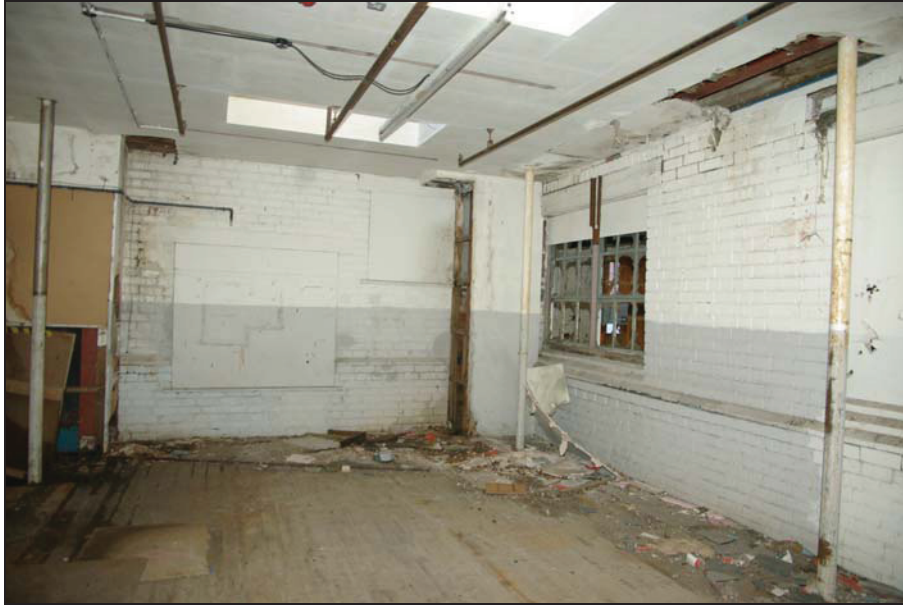
Figure 24. Formerly external walls locating junction between Blocks I and J. Looking south east.
