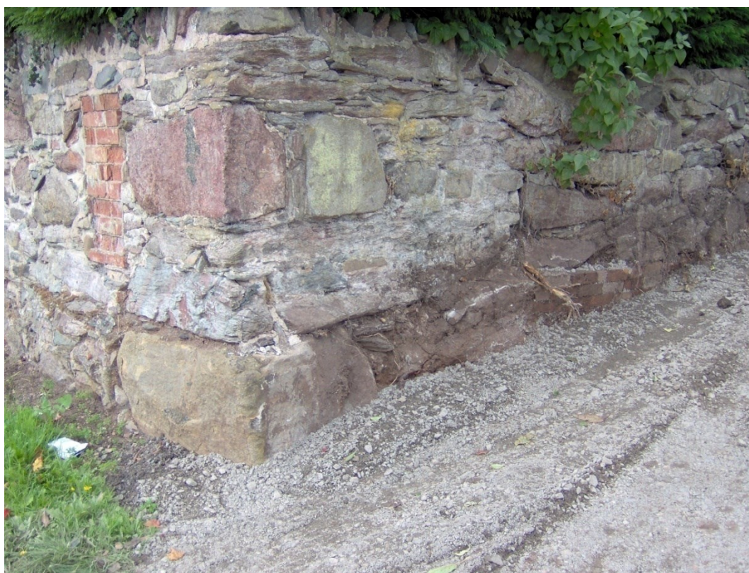
Figure 6: exposed early wall footing on street frontage, possibly the remains of the Post Office building, looking west
