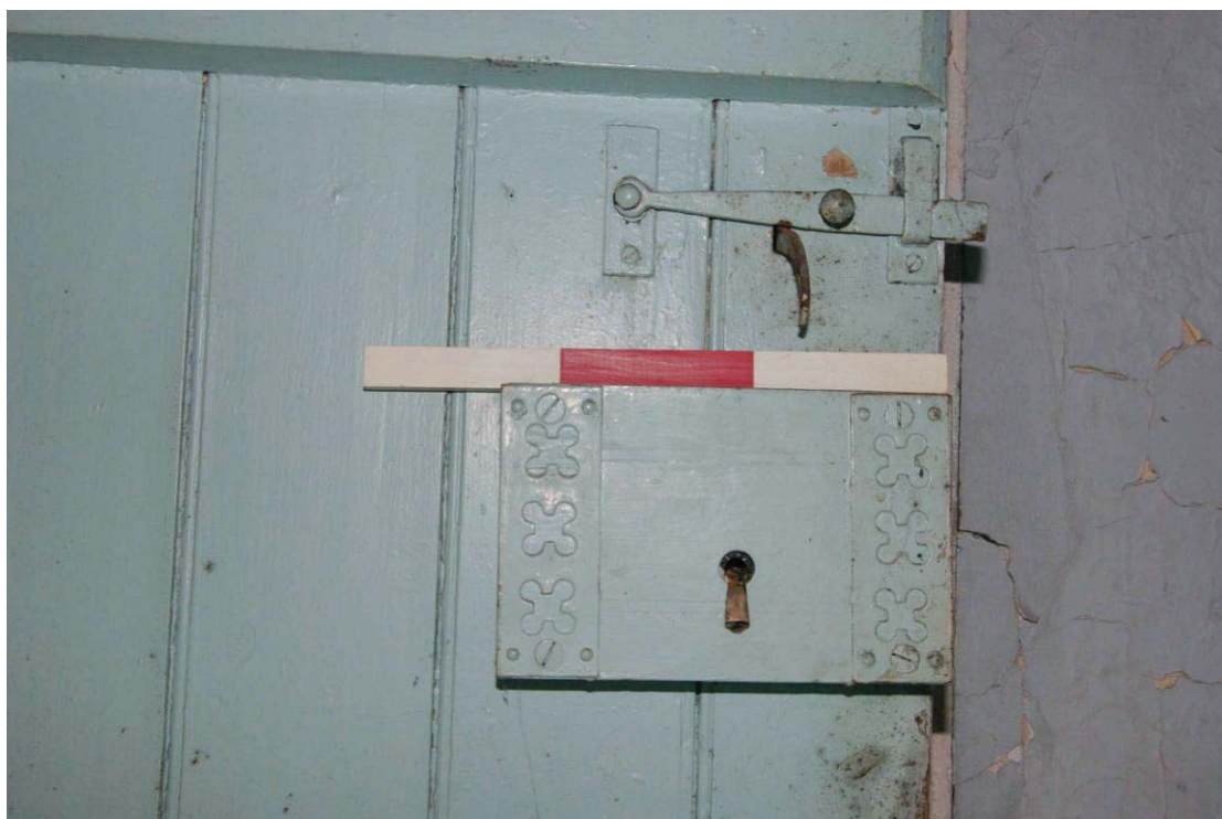
Figure 37 Door to north-east to south-west wing, latch and lock case detail 30cm scale
