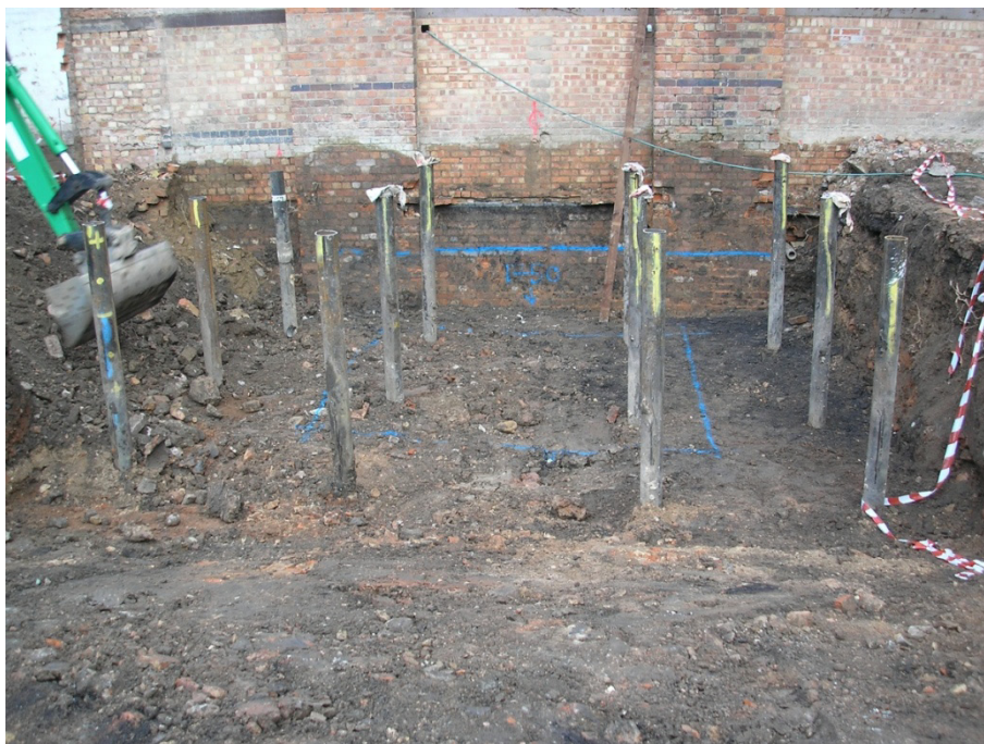
Figure 3: The excavated lift-shaft trench prior to excavation of the internal 2x2m area. Looking north.
