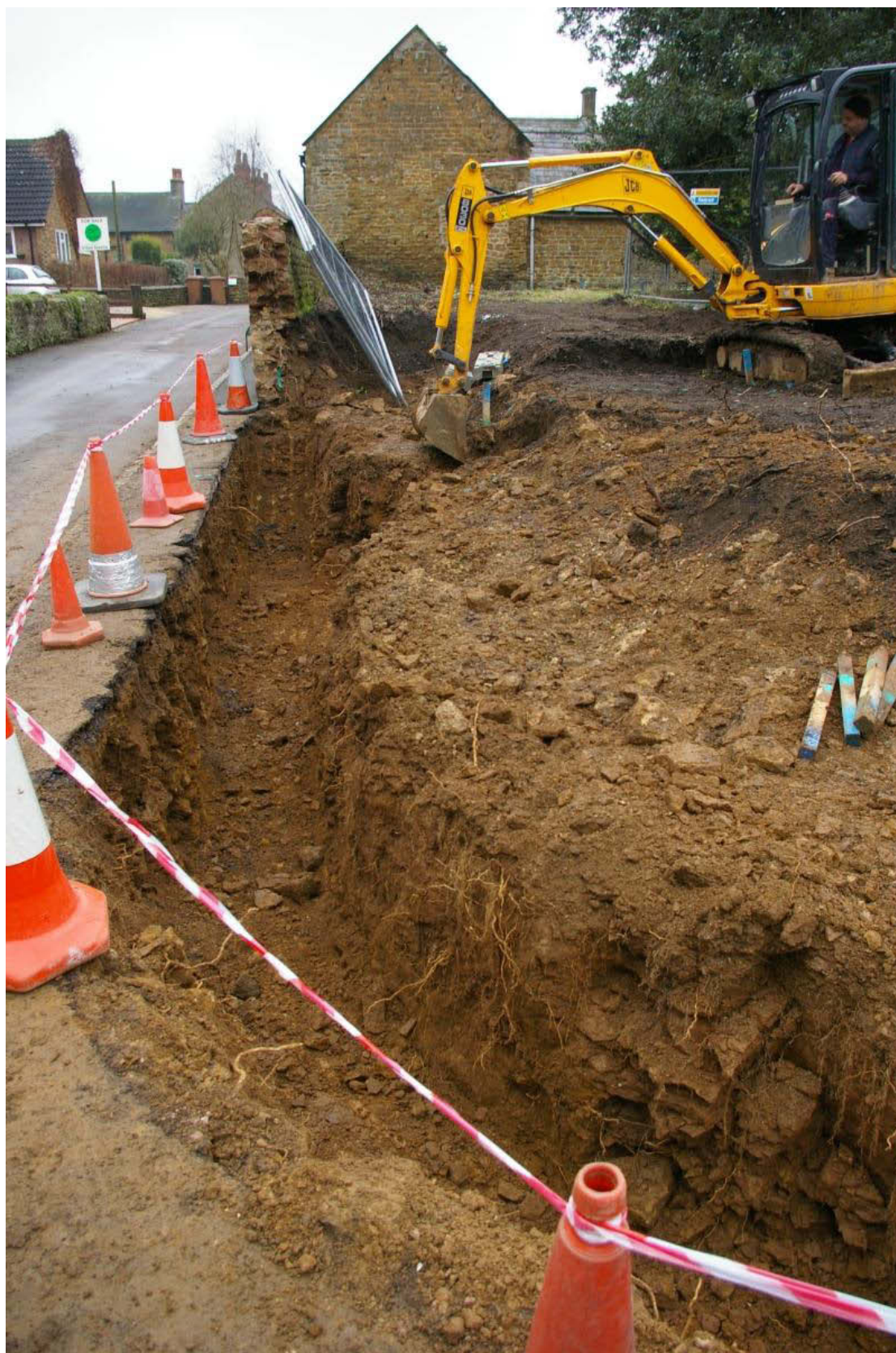
Figure 7 Excavating detached house foundations After demolition of wall and site strip around perimeter of site. Looking north.
