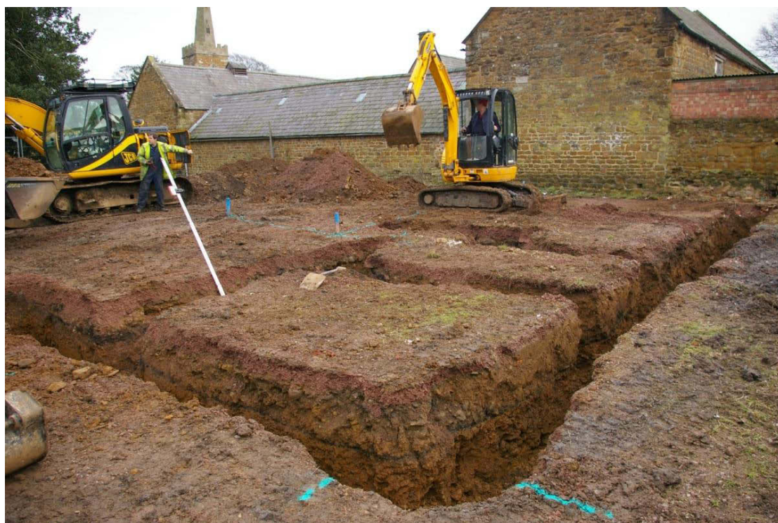
Figure 6 Semi-detached foundations Disturbed upper layers visible above black band of redeposited material. Looking south east.
