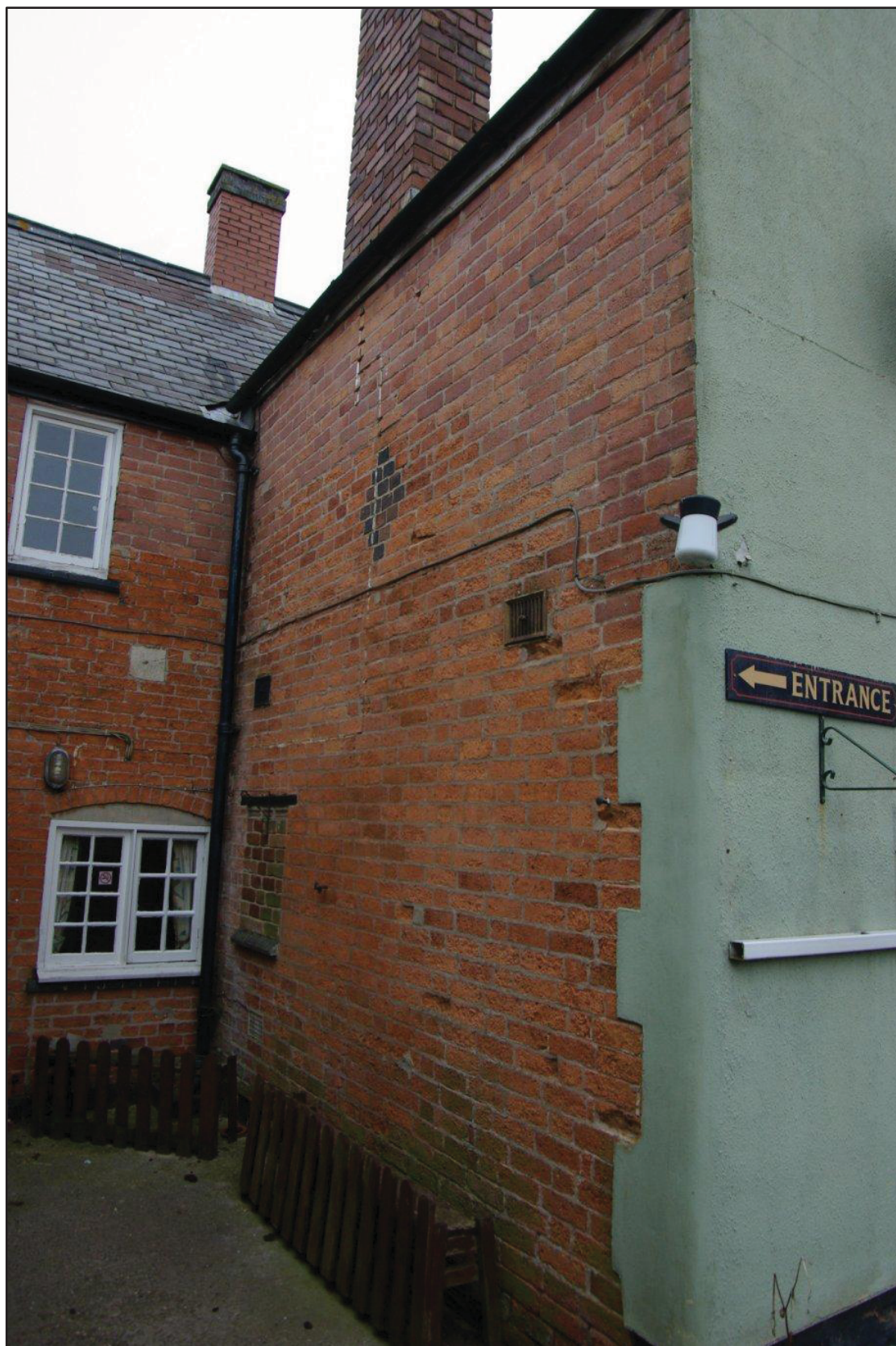
Figure 18 Rear of High Street range and west face of extension Facing north-east
