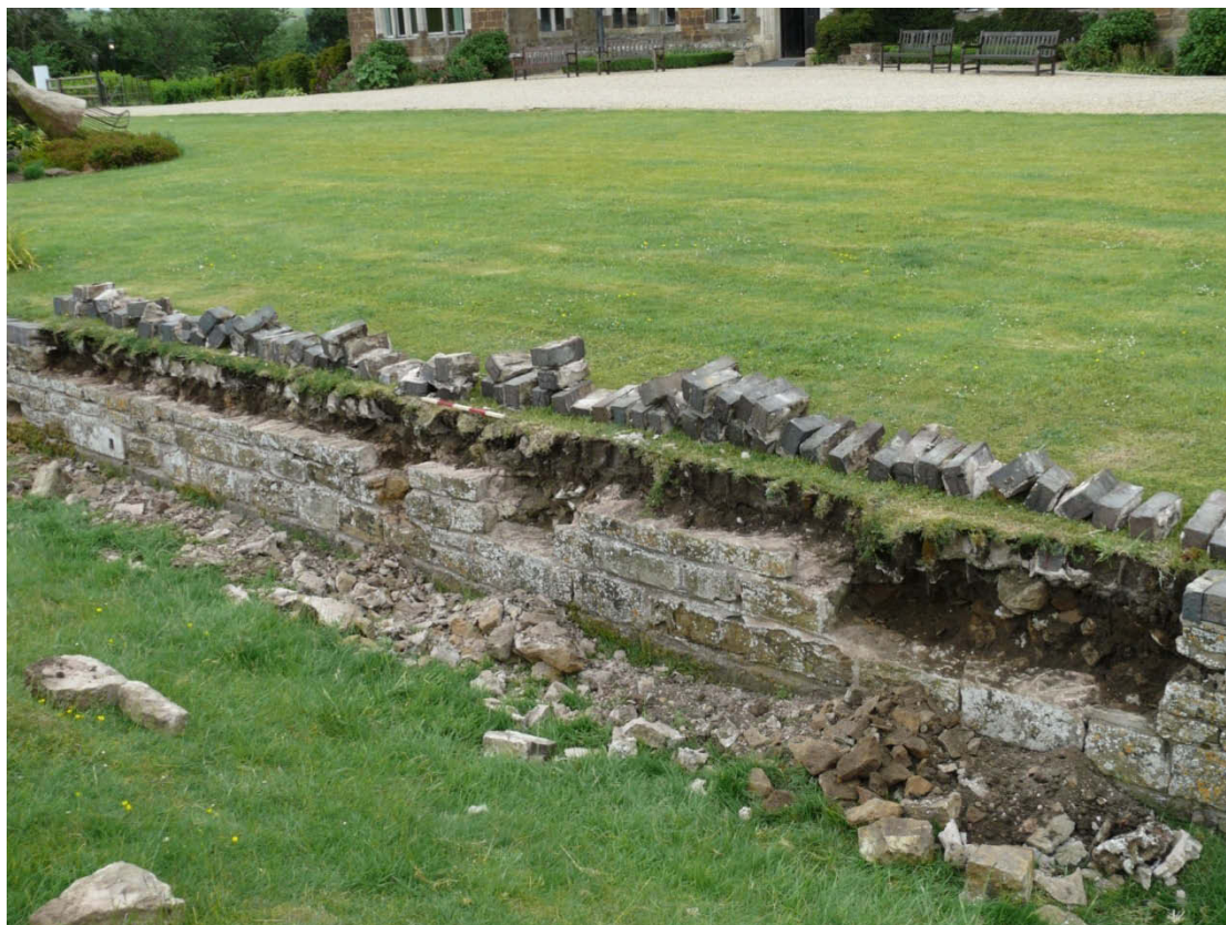
Figure 5 South western portion of Ha-ha after removal of loose stones Facing north east. 50cm scale
