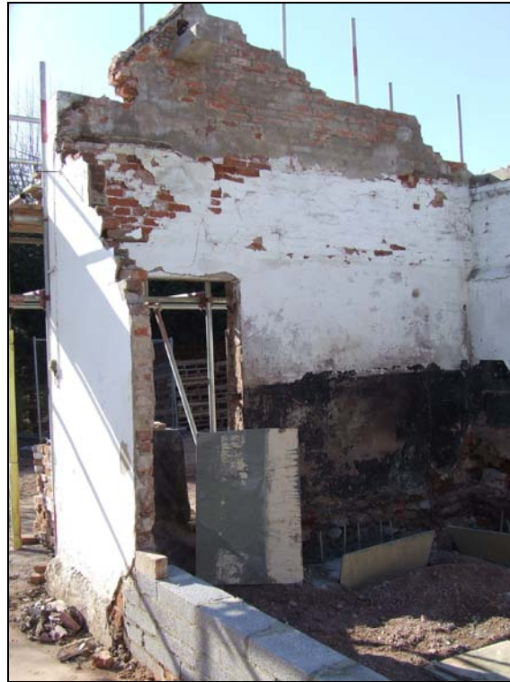
Figure 6 Building from which trusses were removed Note single skin thin brickwork, probably 18th century.
