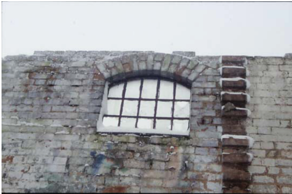
Figure 7 Exposed Iron Framed Window in Rear Wall
