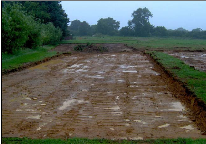
Plate 2 View of footprint of shop after stripping, looking north north-west. Backfilled pond in background
