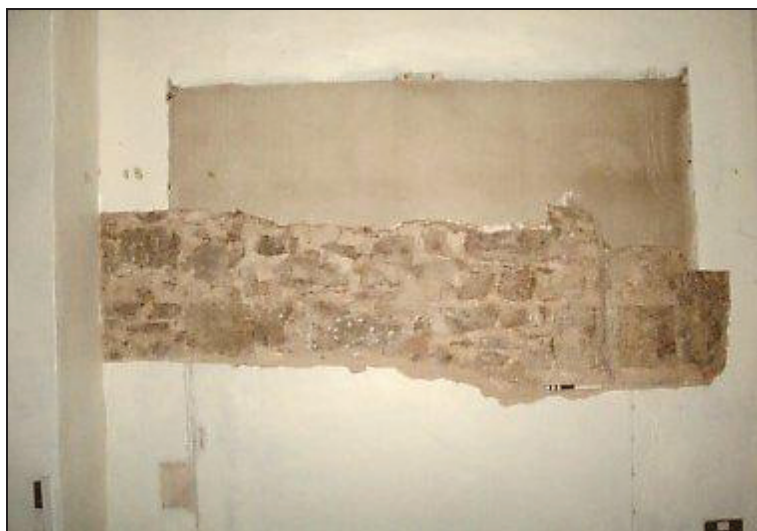
Illustration 4. Opening in plaster on NW wall face, note quoin to right of photo scale.
