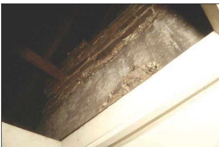
Illustration 6. Rendered stonework above ceiling level on SE wall face, with c. 17th century brickwork above
