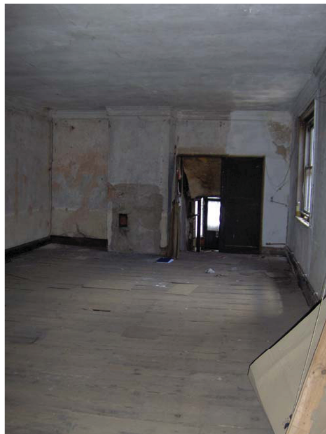
Figure 12: Room G, the long gallery with plaster cornice and chair rail (left of picture).
