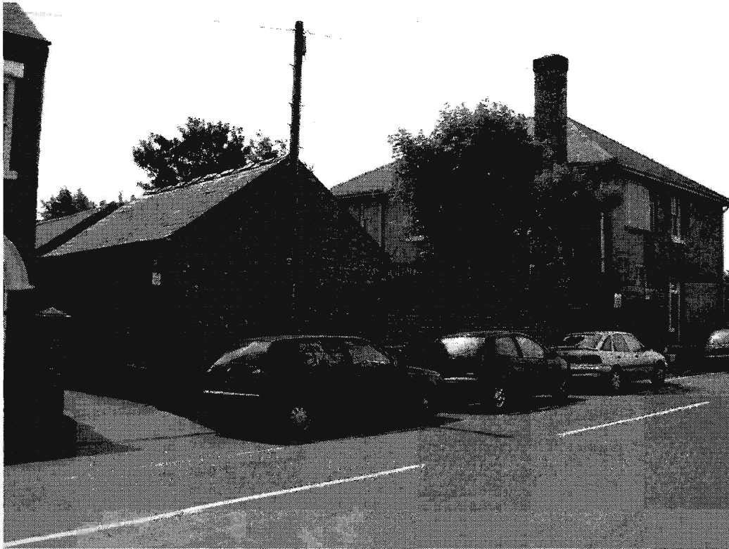
Plate 20. The northern section of boundary wall on Radmoor Road. Note the toothed brickwork into the adjacent courtyard building.
