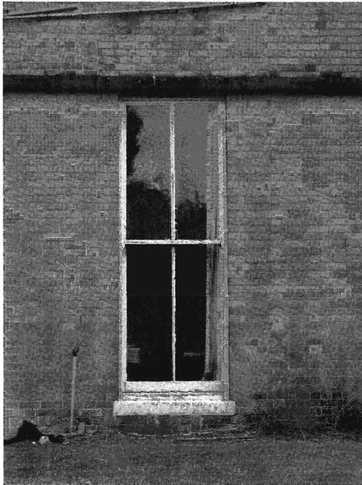
Plate 12. Detail of the full height sliding sash window at ground floor level on the south-west elevation. This window is the first to the left of the bay. Note the stone stringcourse detail above the window.
