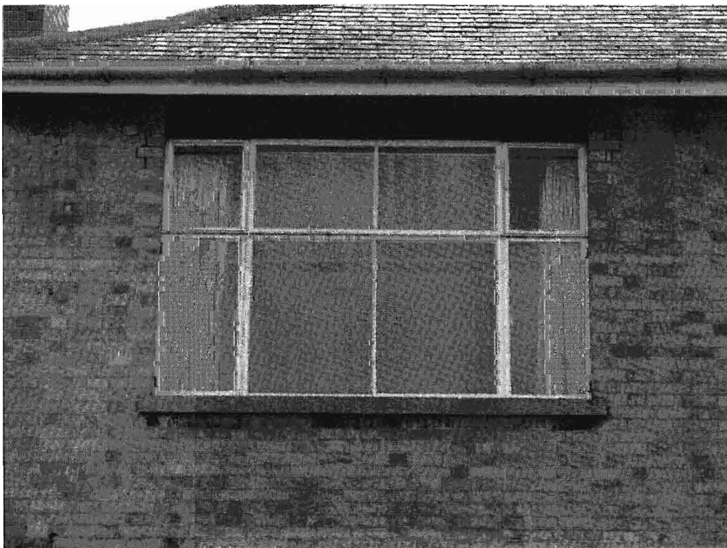
Plate 2. First floor metal framed window on north-west elevation. Note the concrete cill and plain soldier course at the head.
