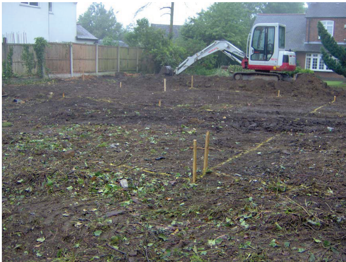
Figure 4 General view showing stripped surface with location of foundation trenches laid out
