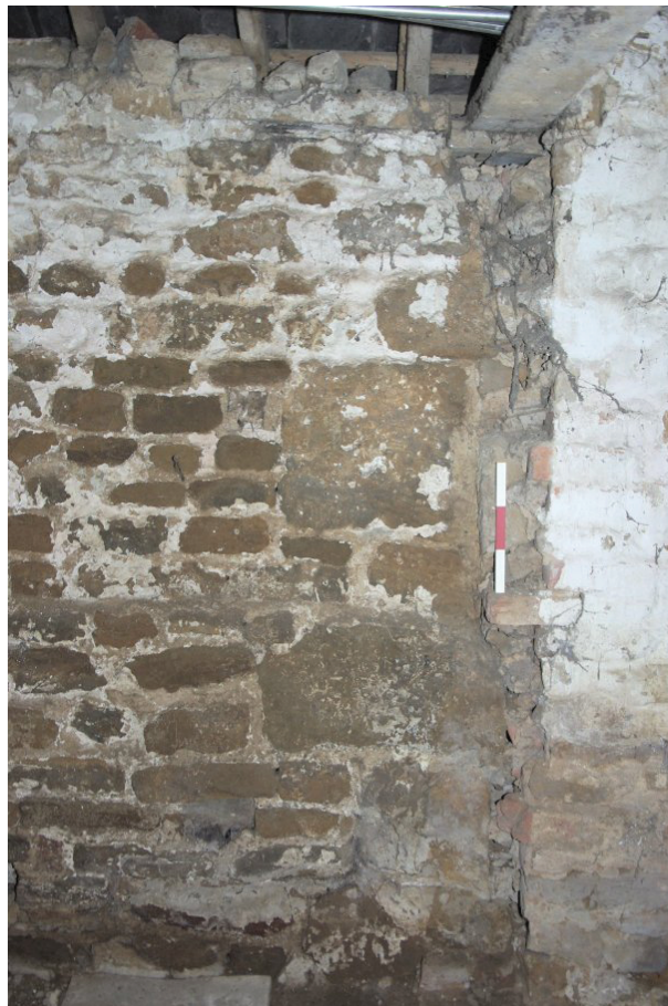
Figure 8 Straight Joint & Quoins in Northern Wall, Bay a .
