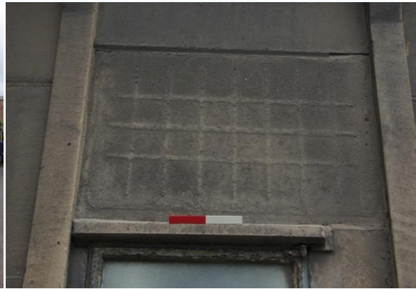
Figure 48 Building 110, detail of alkaline reaction.
