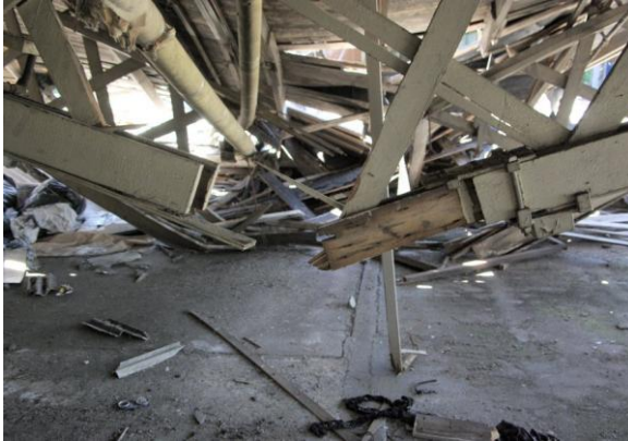
Figure 29 Building 54 Failure in Belfast Truss.
