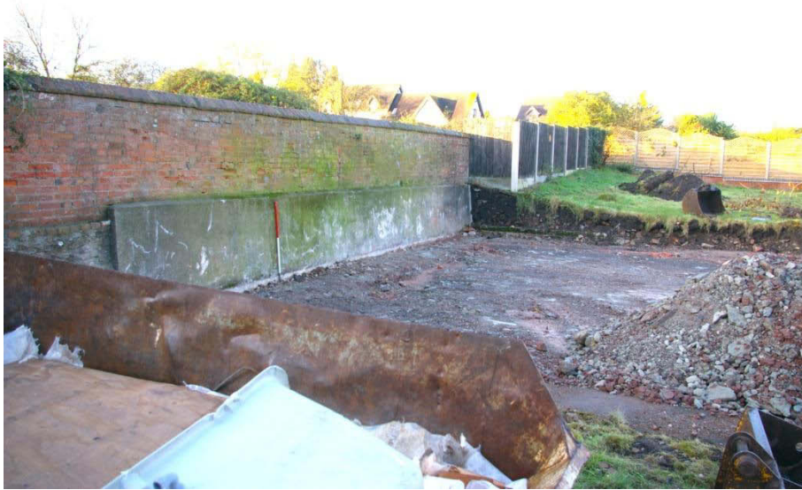
Figure 4 Retaining wall and change in ground level apparent in the southern wall.
