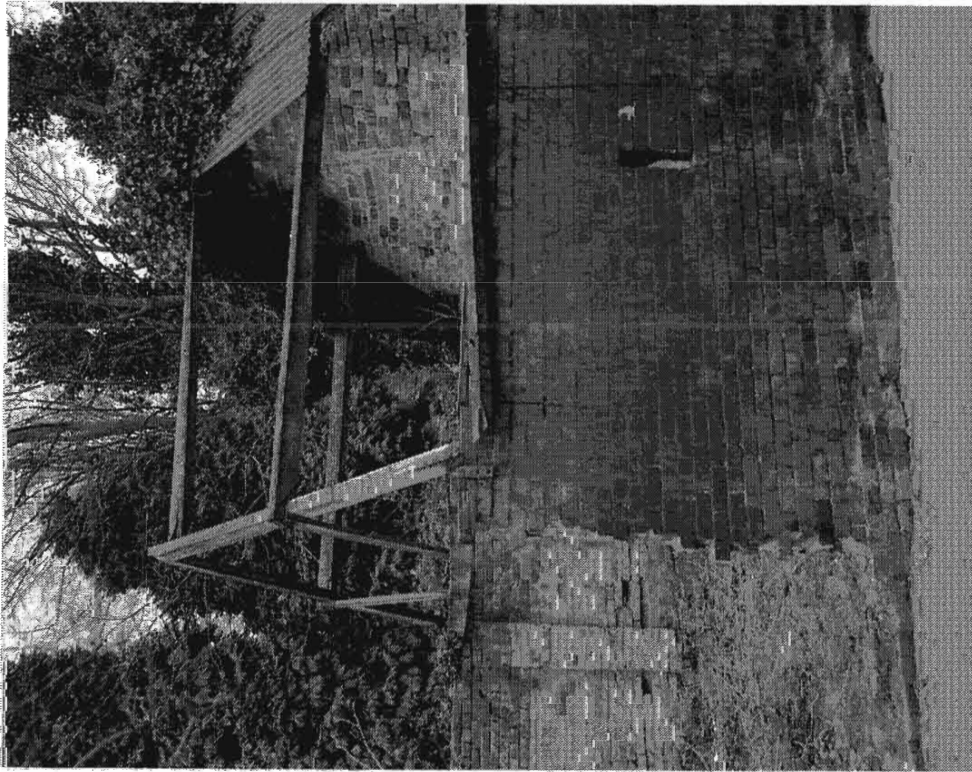
Plate 3 Detail view of side-wall of Bay 2 of the outbuilding showing the only surviving truss set on top of brick piers. The lap jointing of the raked raked struts and the notched joint of the nearside purlin are clearly visible. The end of the metal strap that clasps the tie-beam to the wall-plate and is bolted into the brickwork of the side-wall can also be seen
