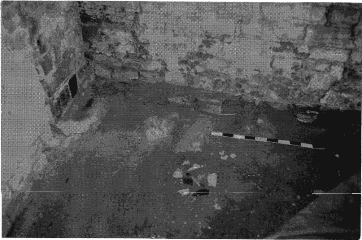
Plate 7 Detail of the base of the rear, brick, boundary wall in Bay 1 showing a base line of stone wall that appears to be all that is left of an earlier stone, boundary wall that has been taken down to provide a base for the present, brick wall and also giving additional space within the building. The base of a large, creamware bowl can be seen trapped in the footings of the stone wall directly above the right-hand end of the scale, other loose sherds of 'Mocha,' pancheon and transfer blue ware are laid out on the floor. The surviving stone footings can be seen underpinning the later, inserted brick work in the first part of the return angle in the top left of the photograph.
