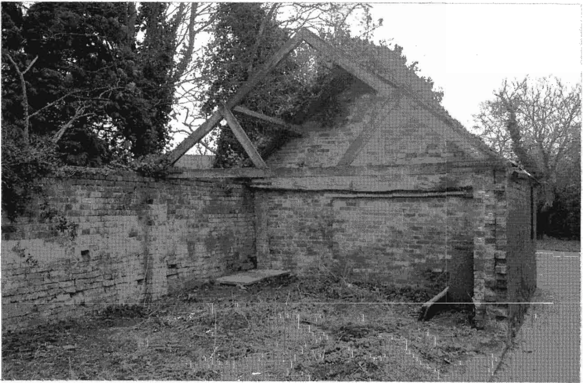
Plate 9 General view of the ruinous condition of Bay 2 of the Outbuilding, looking from the north-west and showing the single, surviving deal, truss and the rear, brick boundary wall with the Churchyard behind. Also shows a large, hardwood beam spanning the bay close to the transverse wall between Bays 1 and 2.
