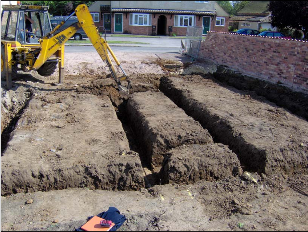
Figure 5. Trenches nearing completion. Concrete capping for well near to the Heras fencing top right.
