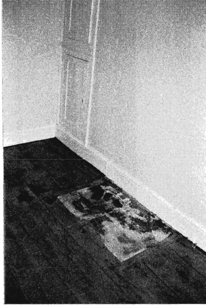
Plate 47 Hearth of removed fireplace in second floor, north wall of 19 th century build.
