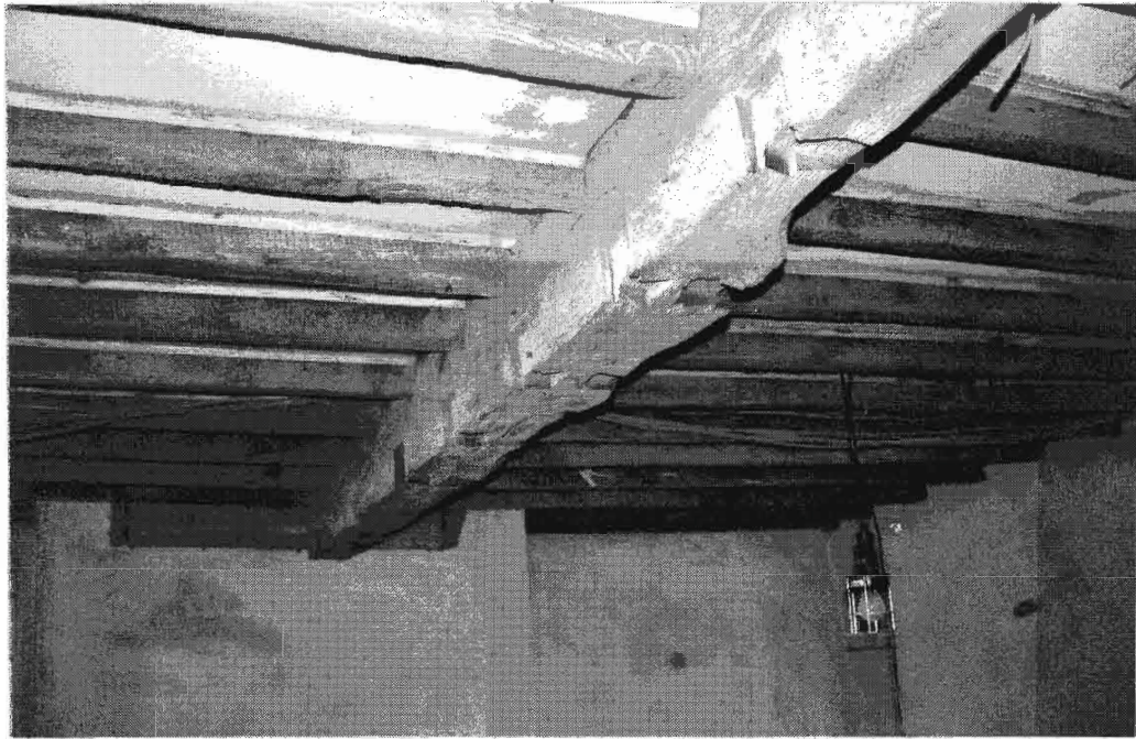
Plates 25 Detail of ceiling structure at first floor showing re-used beam and joists.
