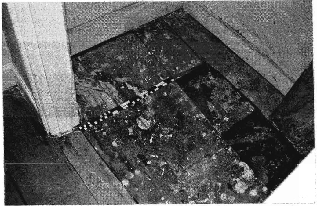
Plate 41 Wide hardwood floorboarding exposed in cupboard under stairs of 19 th century first floor.
