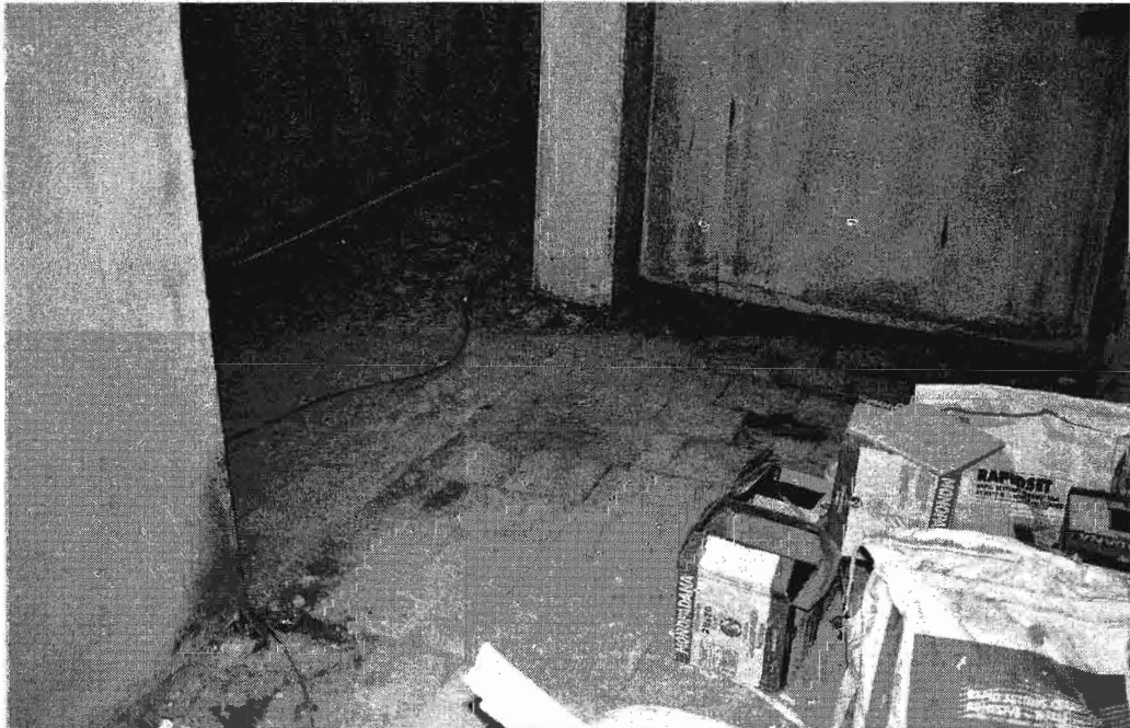
Plate 26 19 th century quarry tile and brick flooring in 18 th century part of building.
