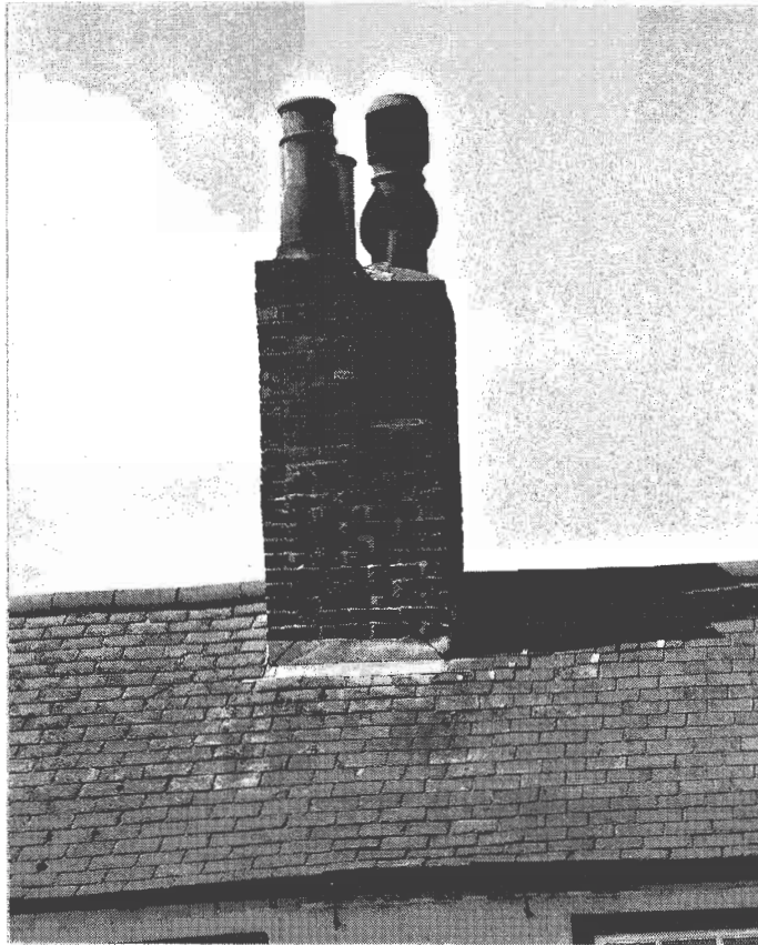
Plate 5 (above) detail of altered chimney stack in 18 th century part of building, also shows Welsh slate roof, also shows dentil course of brickwork at eaves.
