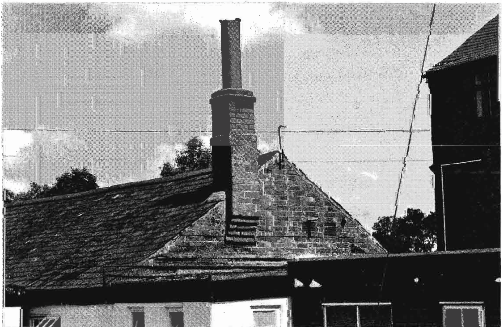
Plate 18 (below) view from south-west showing pitched Welsh slate roof and gable chimney to single-storey converted farm building.
