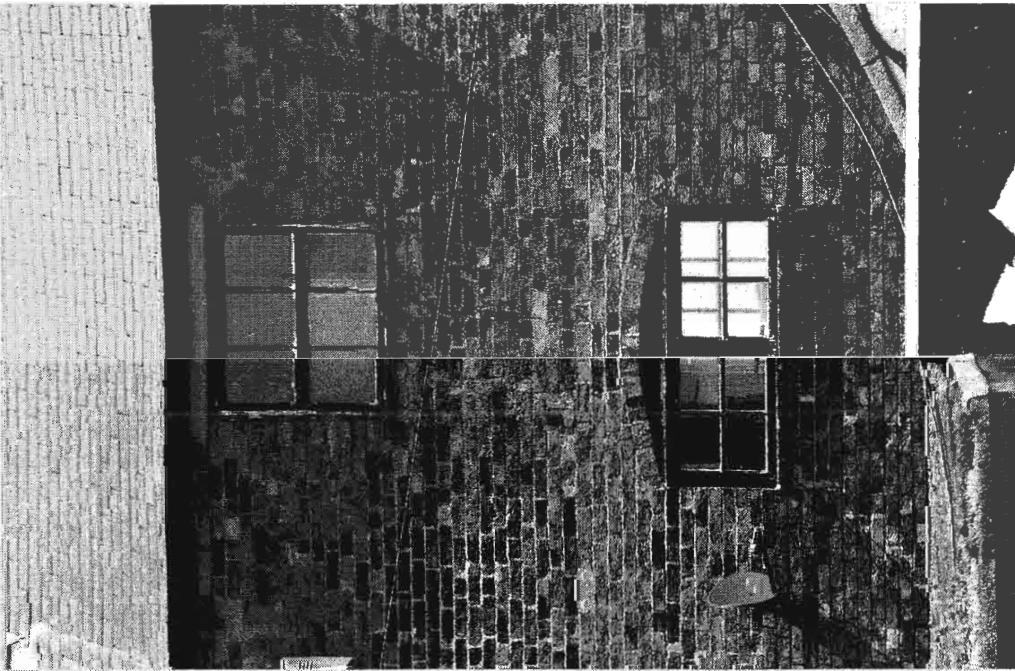
Plate 15 Detail of 19 th century building's west elevation, showing three-over-three paned, sash window at second floor and segmental arched window at first floor. Also shows Flemish garden Wall Bond of this elevation. The gable palimpsest, part of which can be seen in this photograph appears to be part of a now demolished building shown on early Ordnance Survey maps.
