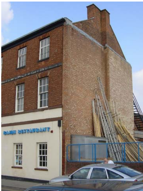
Figure 1: Grade II listed No.59 Highcross Street. Note the 'skin' wall against the southern gable end.
