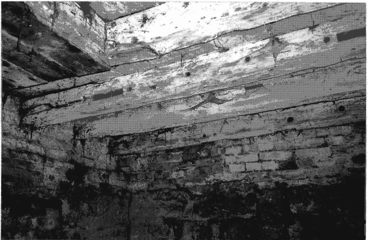
Plate 4 Detail showing joists to floor of room G 1 in cellar with vee-grooves, mortises and stale holes, being re-used sections from a timber-framed building.
