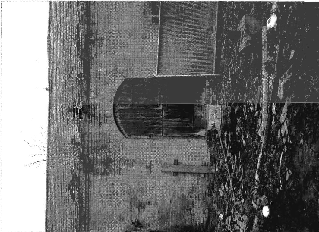
Plate 15 Front elevation detail of Barn B, showing the single, wagon entrance door with arched head. Detail of the eaves brickwork is visible where the roof tiles have slipped.
