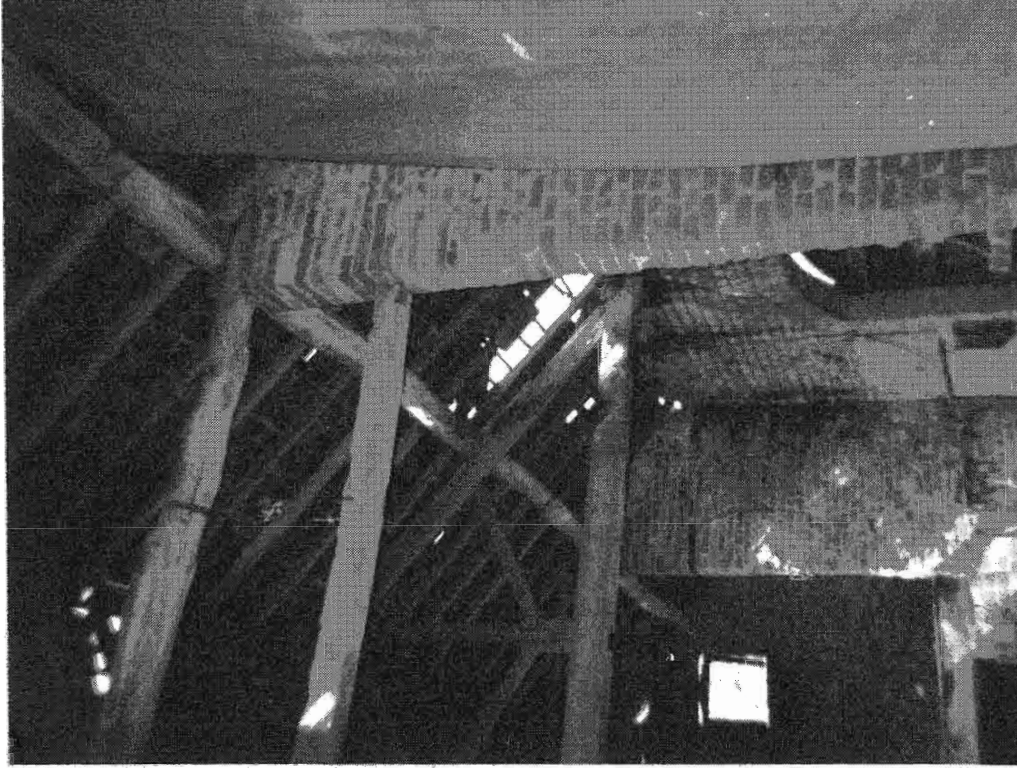
Plate 16 Interior detail of Barn B showing the brick flank walls at the wagon entrance bay and single, king-post roof truss.
