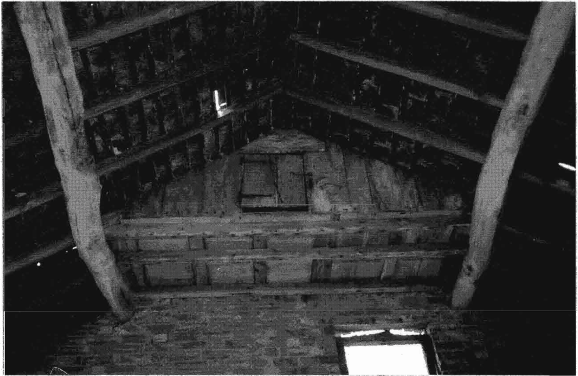
Plate 19 View of the late, C18 pigeon loft, supported by the topside of the purlins and set in the apex of the south gable of Barn B.
