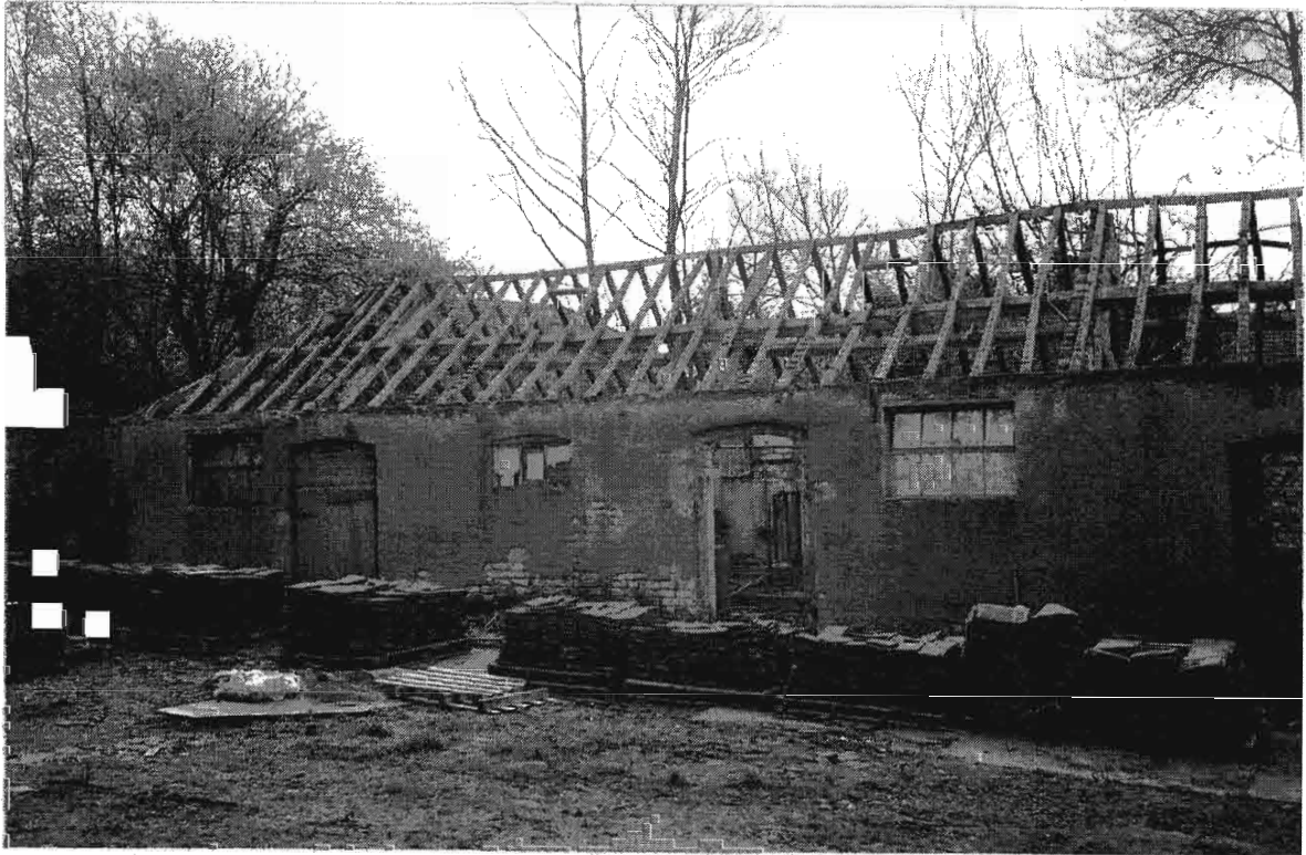
Plate 13 General view of part of Barn A, showing hipped gable at its west end and conventional type of windows and doors present.
