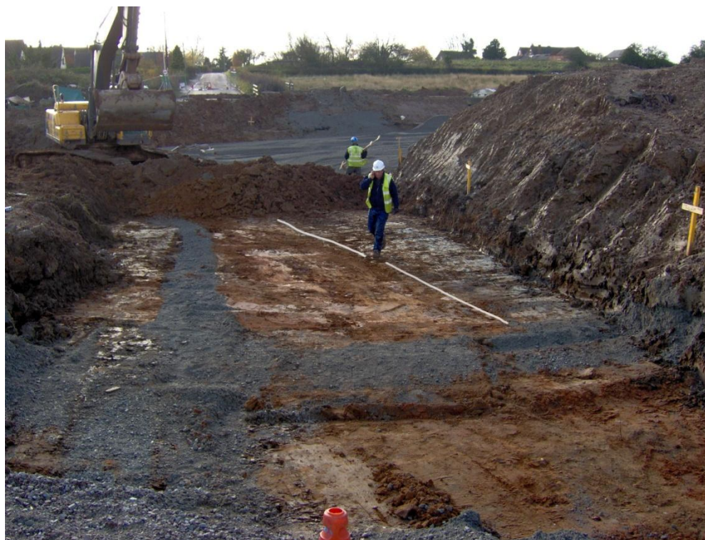
Plate 2 Site 4, removing the Station Road carriageway (11/11/08), looking south. Edge of pond material highlighted.
