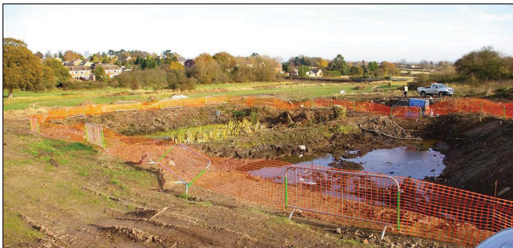
Plate 7 The ponds after clearance and removal of modern landfill, looking north-east. Foreground Pond 3 (flooded), left Pond 1.
