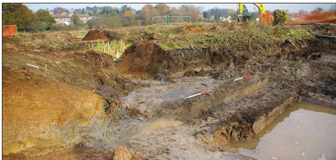
Plate 8 Pond 3 during machine excavation, showing sections through banks and partition and depth of fill. Looking north-east
