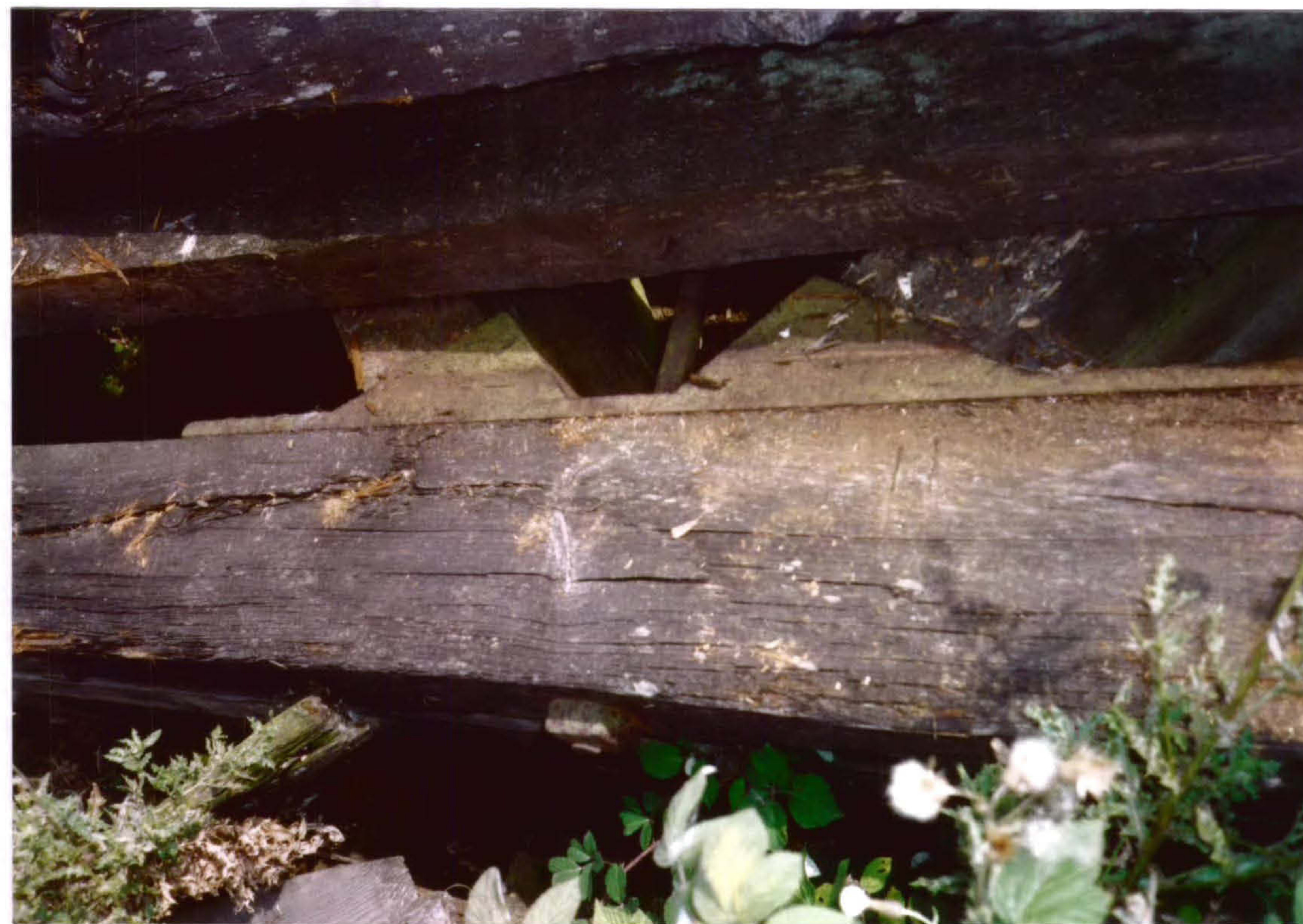
Plate 14 Detail showing a cast-iron show for raked struts set onto the tie-beam of a principal rafter truss. The lower part of the bolt passing through the tie-beam and rising to the cast iron housing at the truss apex can also be seen, as can a carpenter's construction mark II. (Timber dump)
