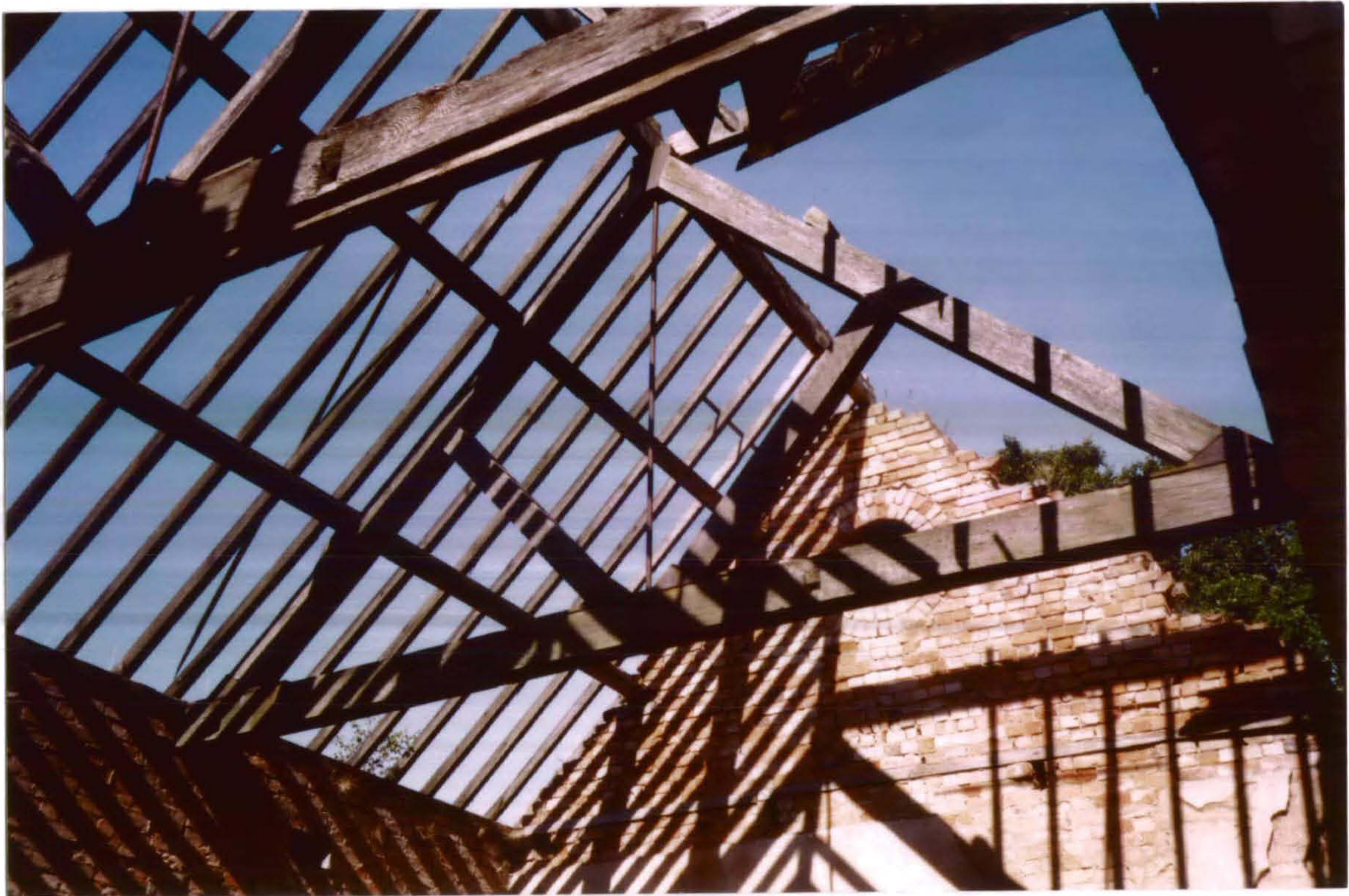
Plate 32 West Range Internal – north-west corner of range. Bolted principal rafter truss with cast-iron shoe for the base of the raked struts and cast-iron apex junction, October 2003, now removed. A wooden bonding course can be spanning the full width of the bay at the base of the gable brickwork. (see Drawing 8)
