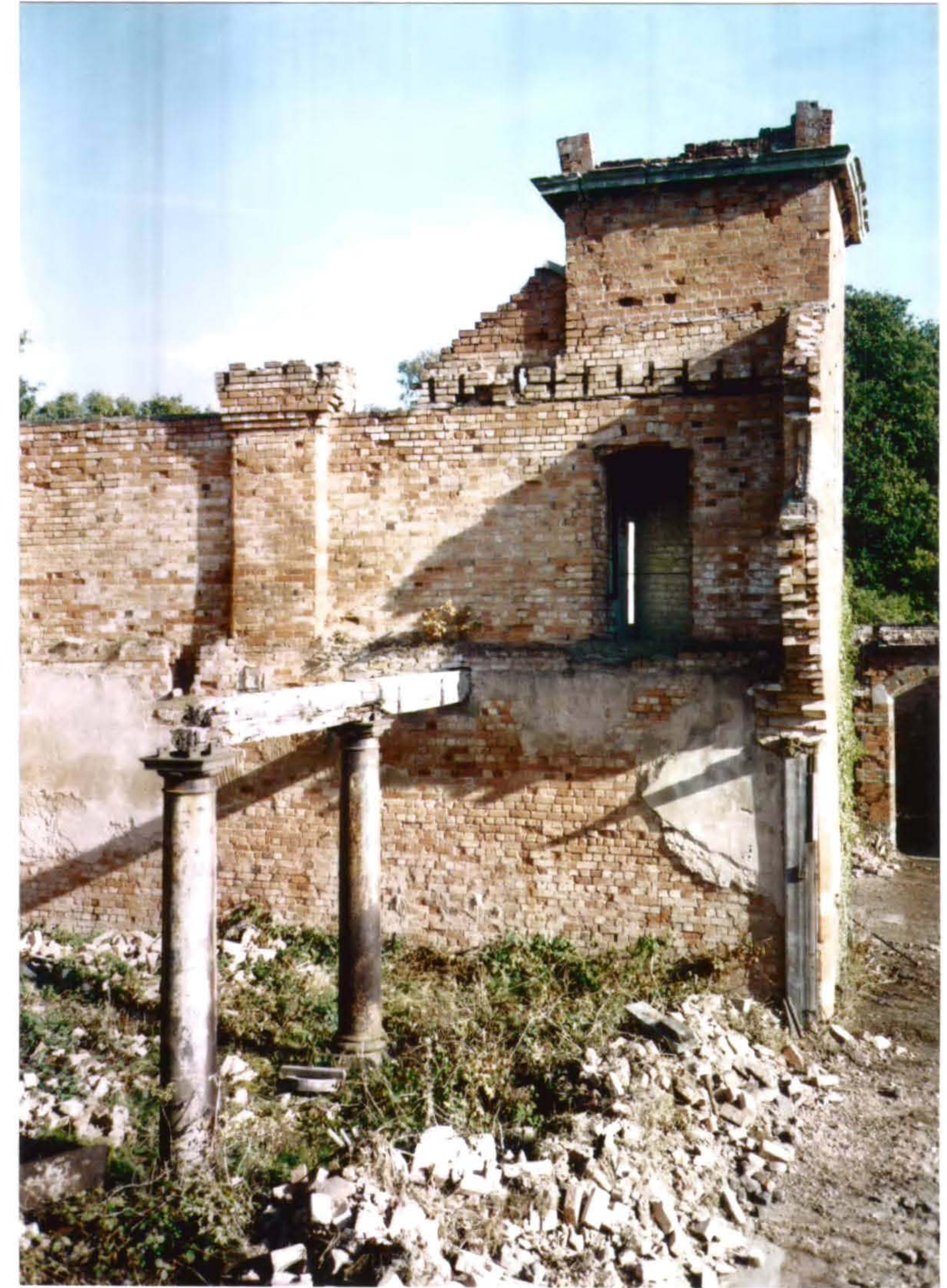
Plate 36 Shows the surviving pair of cast-iron columns with the floor beam pocketed into the north-east wall of the Carriage House and first floor access from the stair tower.
