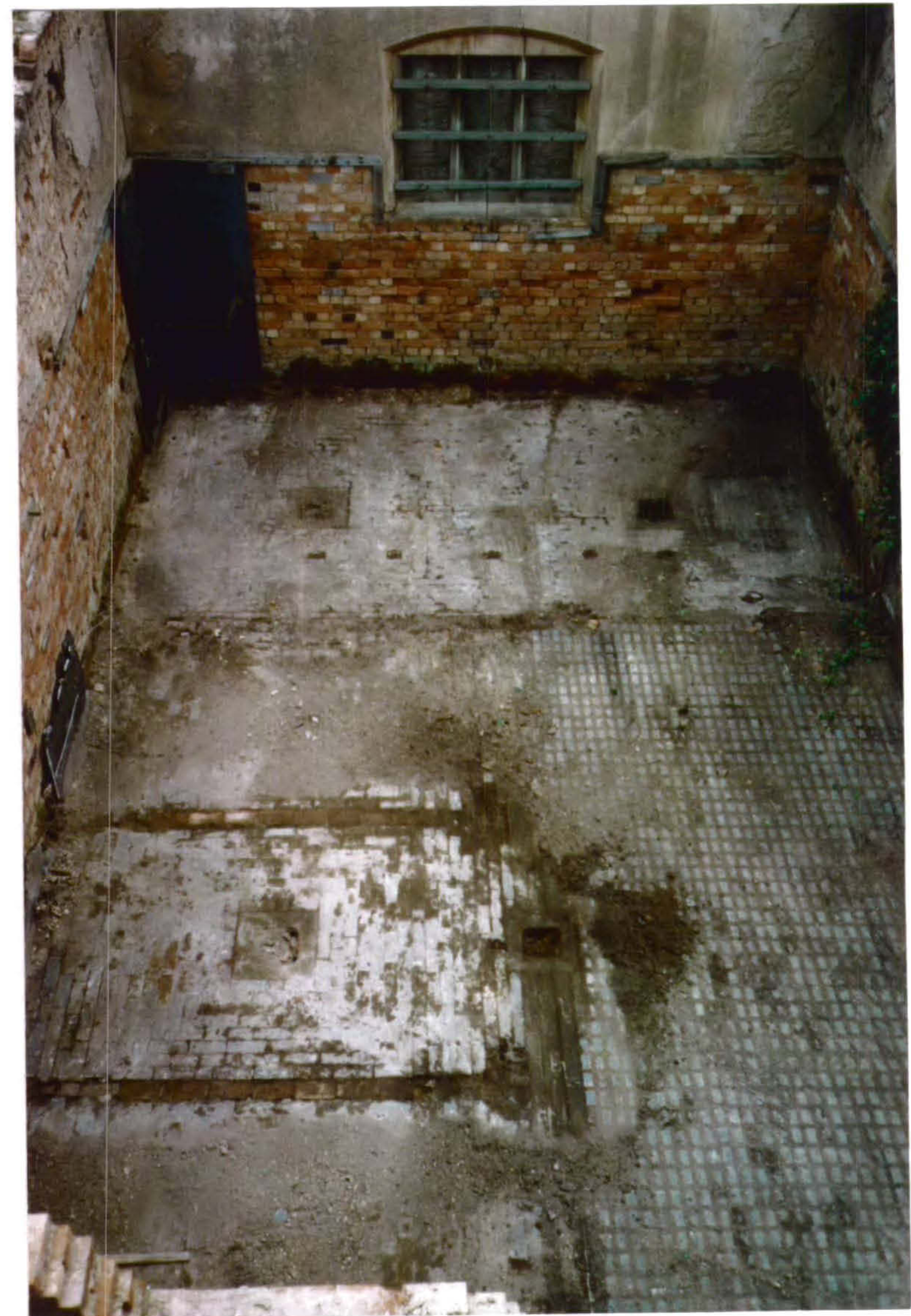
Plate 44 East Range Internal - south-east corner of range showing layout roof of Stabling for five hunters. The window is in south-east gable of the South Elevation.
