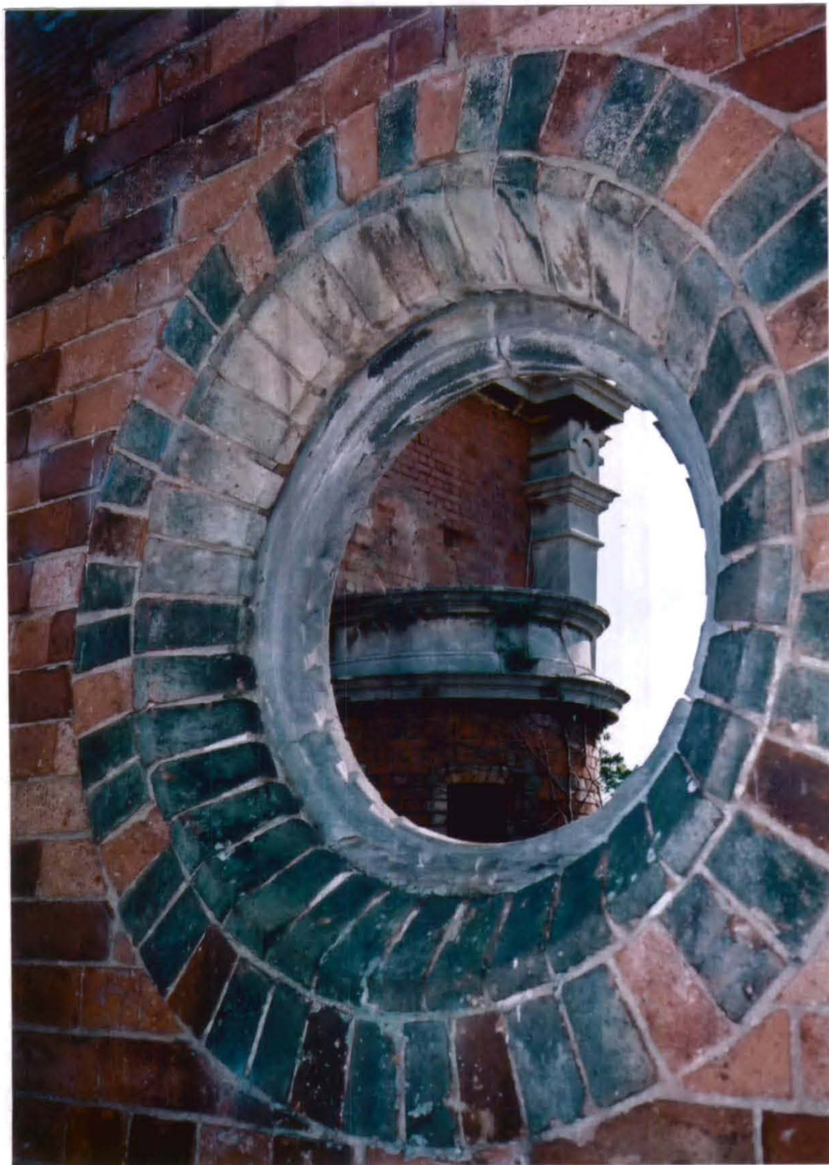
Plate 21 Detail of large oculus with chamfered brick surround and wooden window base. The stone surround at the top of the Clock Tower, Stair Tower is visible through the opening. The scarring of the Clock Tower brickwork relates to the original cupola of the Stair Tower. (South Range Interior)
