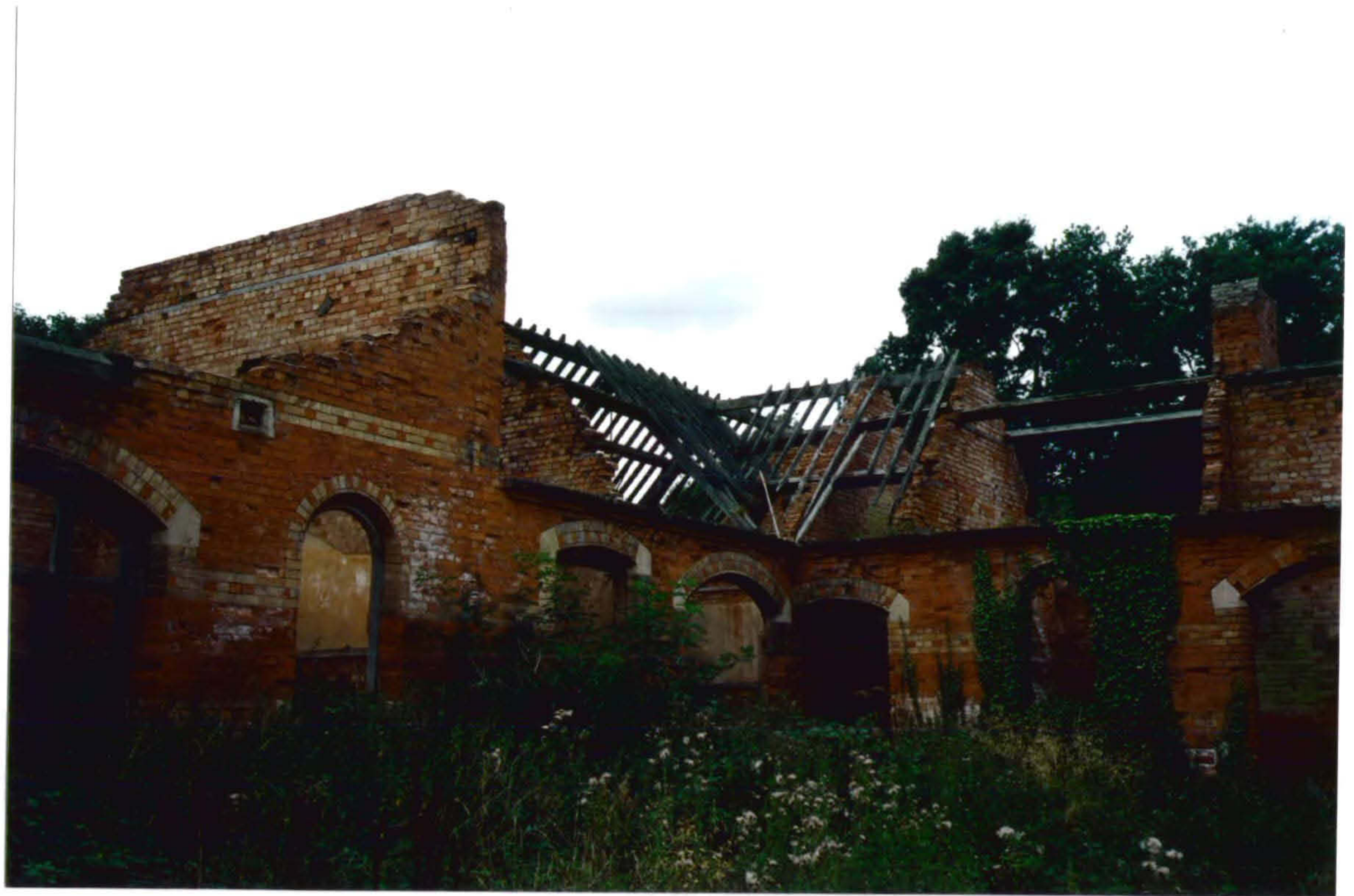
Plate 33 West Range, north-west corner, showing roof frame intact and roof section over rear passageway, October 2003, roof timbers removed 2004.
