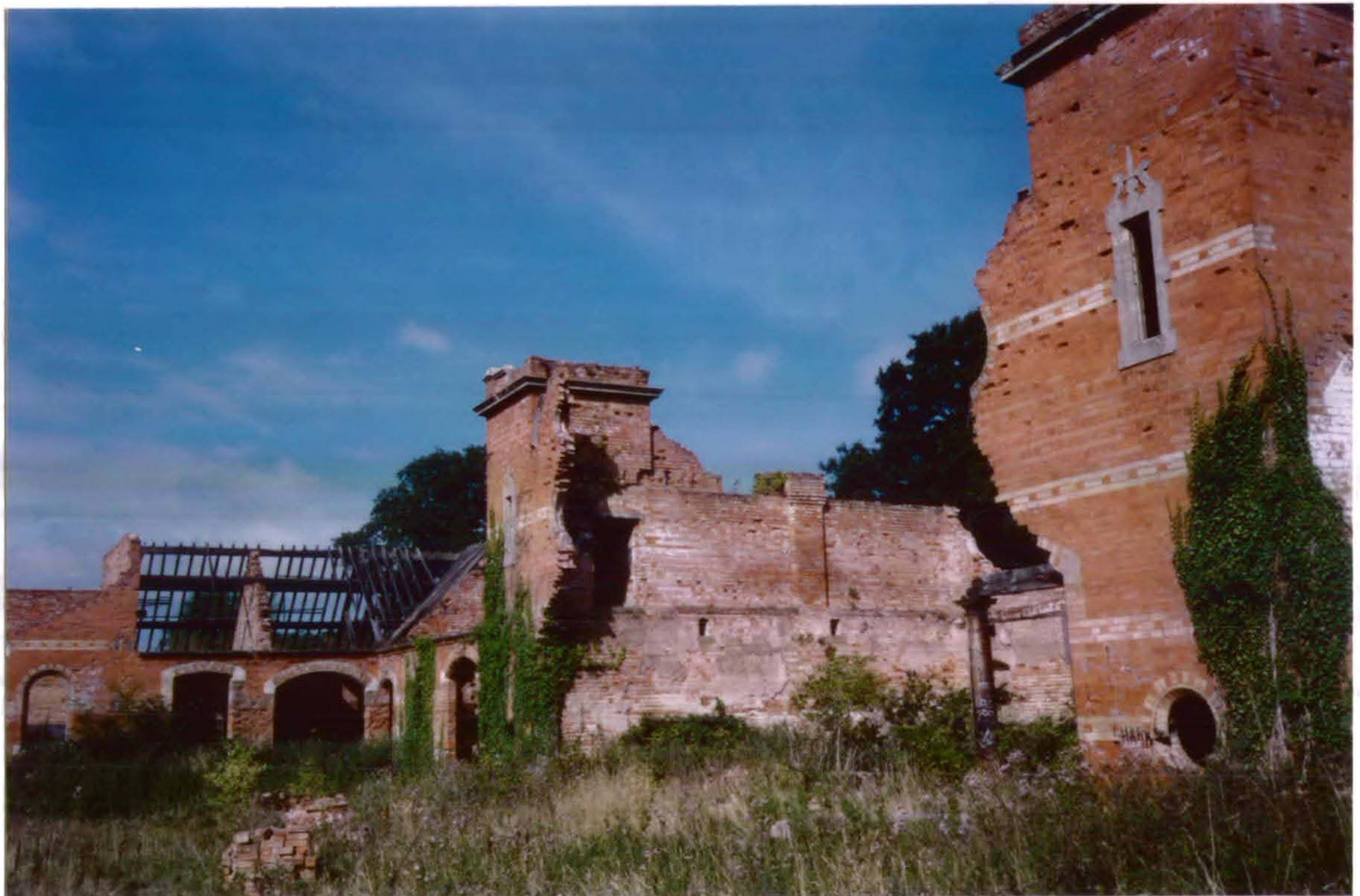
Plate 34 North Range – general view towards the West Range, showing the void where the Carriage House entrances stood.
