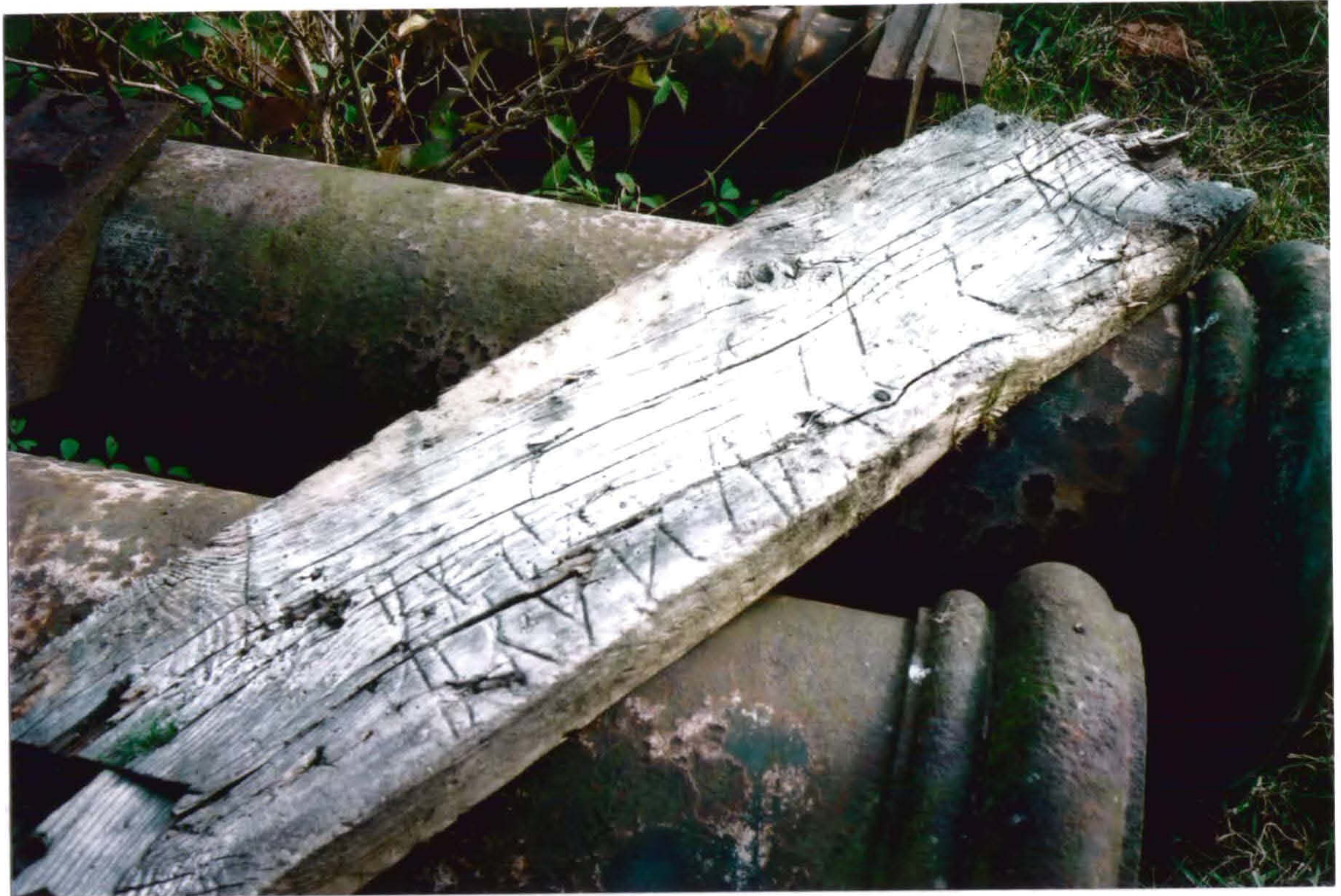
Plate 11 Timber section with rase markings, see Fig.iii, p.26. The beam is sitting on top of two cast-iron columns similar to the two surviving examples standing in the Carriage House area. Location: salvaged materials area.
