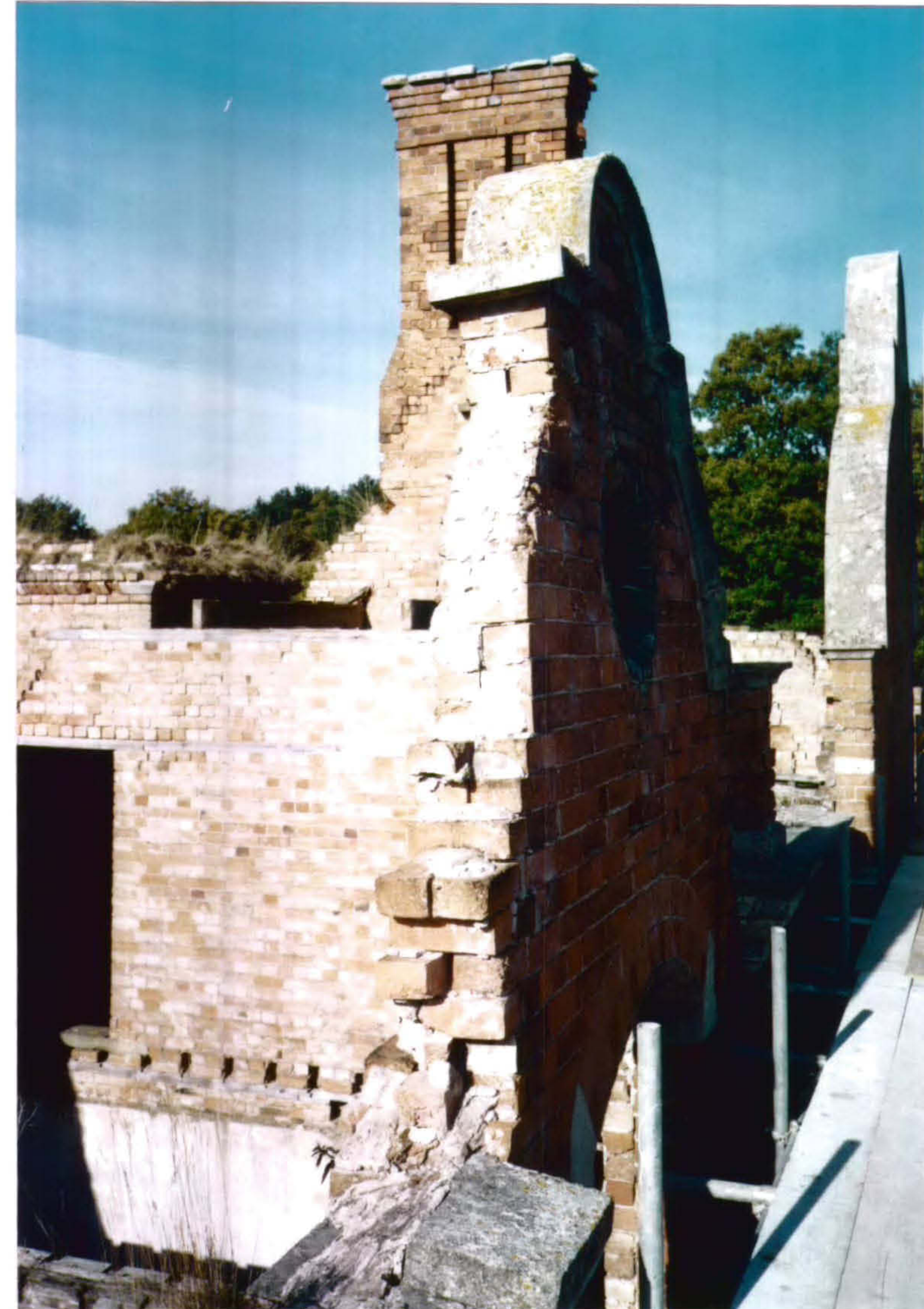
Plate 28 West Range – small Dutch gable structure weakened by weathering and general deterioration of the fabric.
