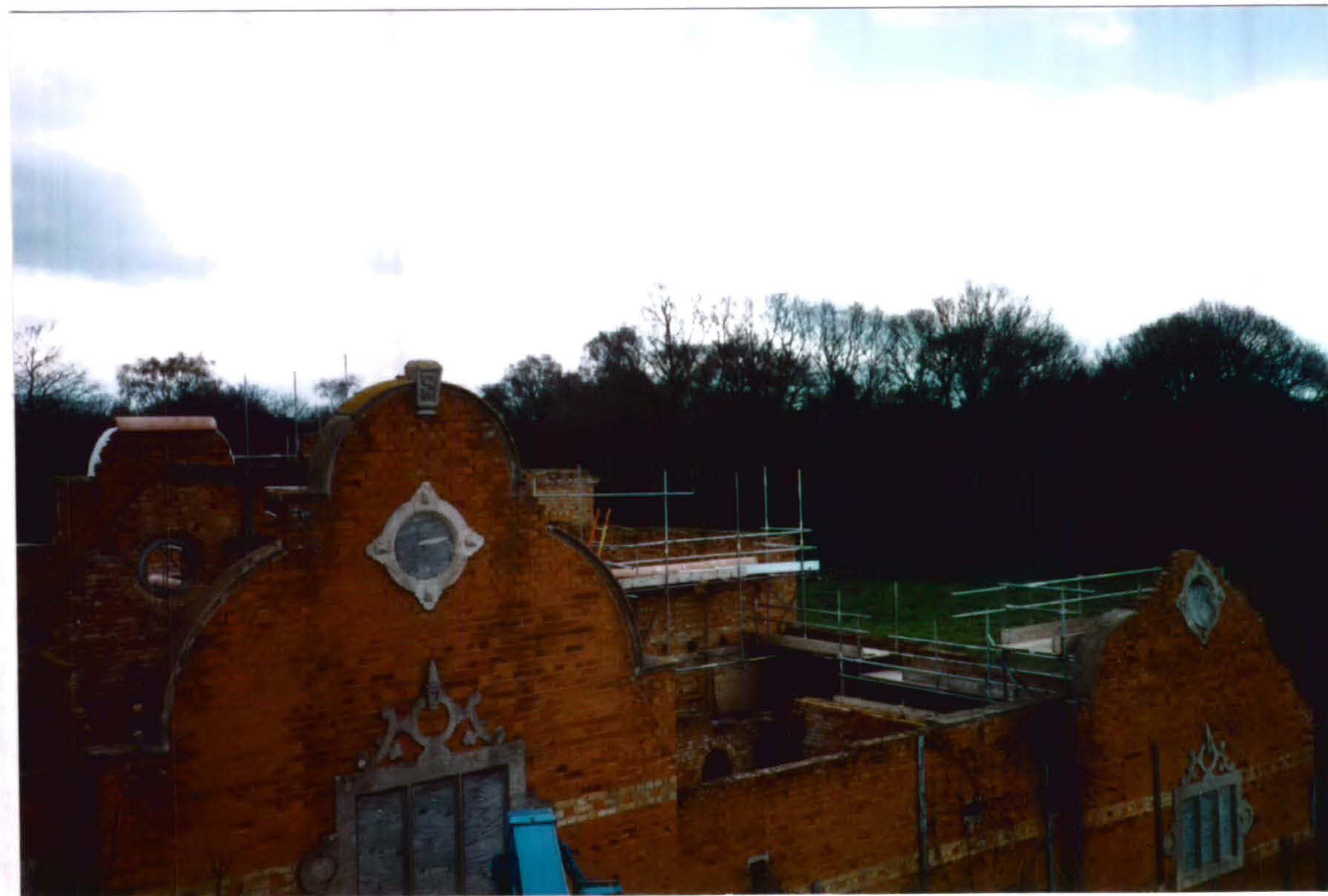
Plate 18 South-east section of South Elevation. The rear Dutch Gable has the ceramic coving installed that is part of the 'conservation' programme undertaken during 2003-2005.
