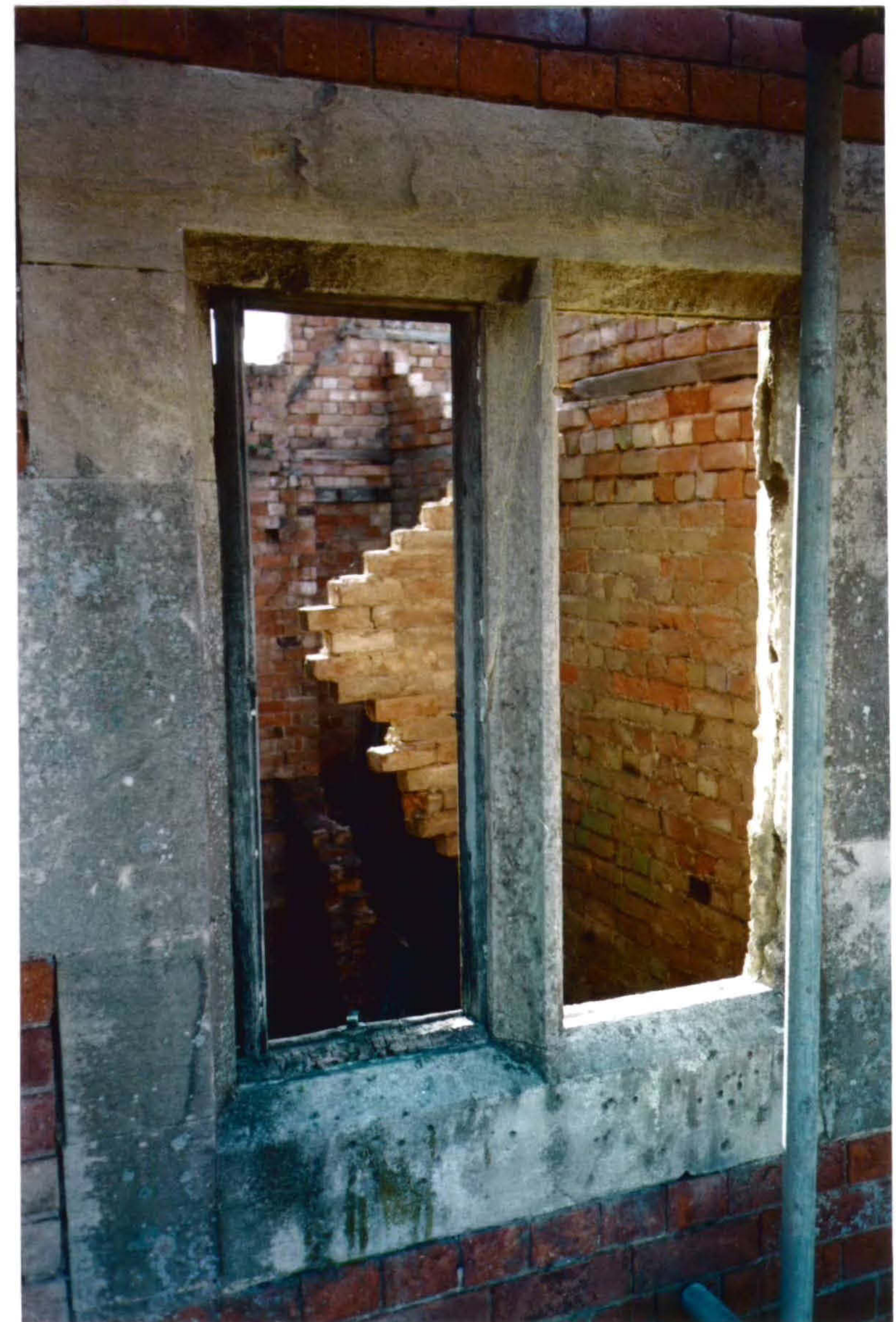
Plate 6 Detail showing two-light, mullion window with wooden a surviving wooden frame still in position on South Interior.
