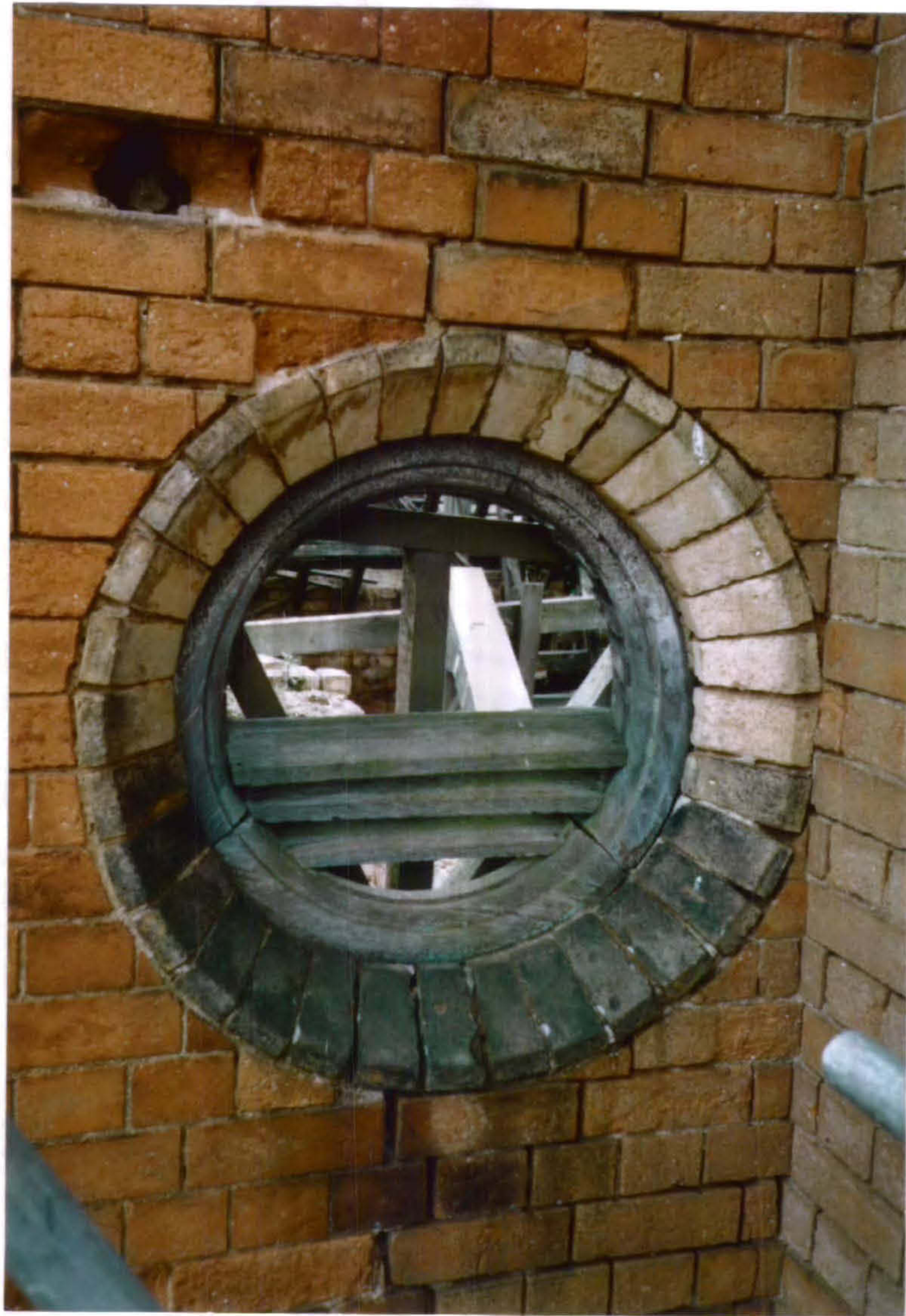
Plate 3 Detail showing chamfered bricks forming a small oculus in the brickwork of the South Range Interior.
