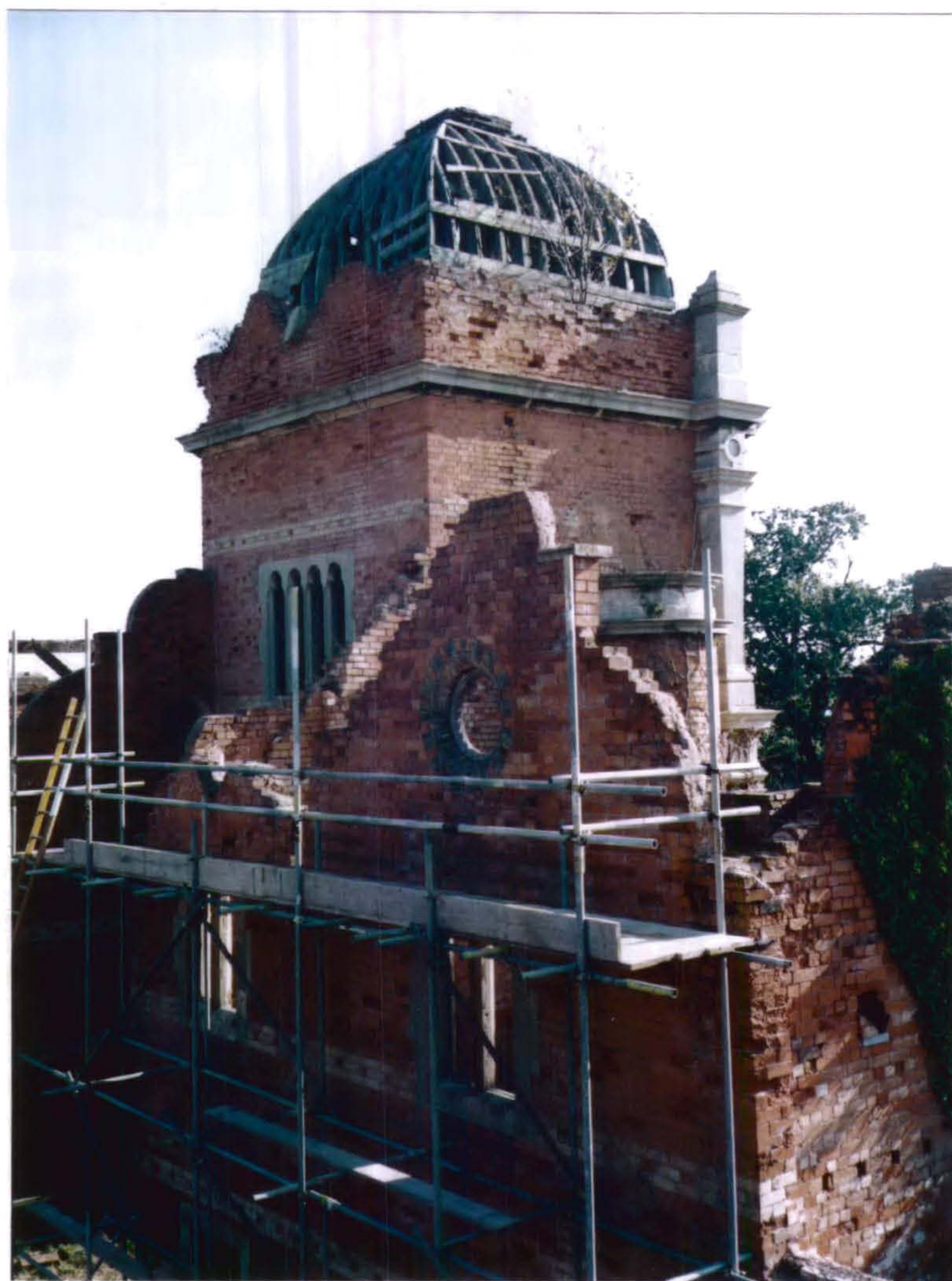
Plate 19 South Range Interior - General view across to Clock Tower from Stable Yard, showing the exposed framework of the cupola.
