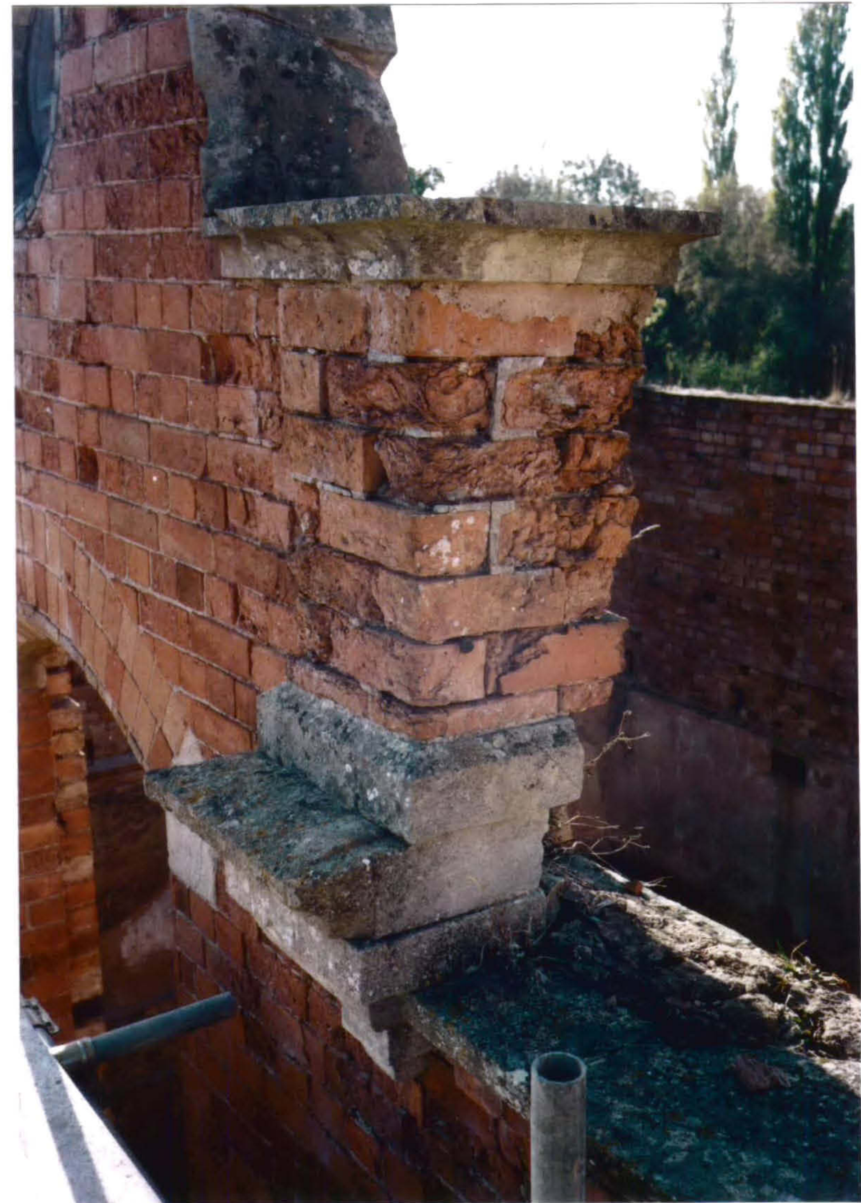
Plate 26 West Range Interior showing derioration of brick fabric and stone coping weakened by weathering.
