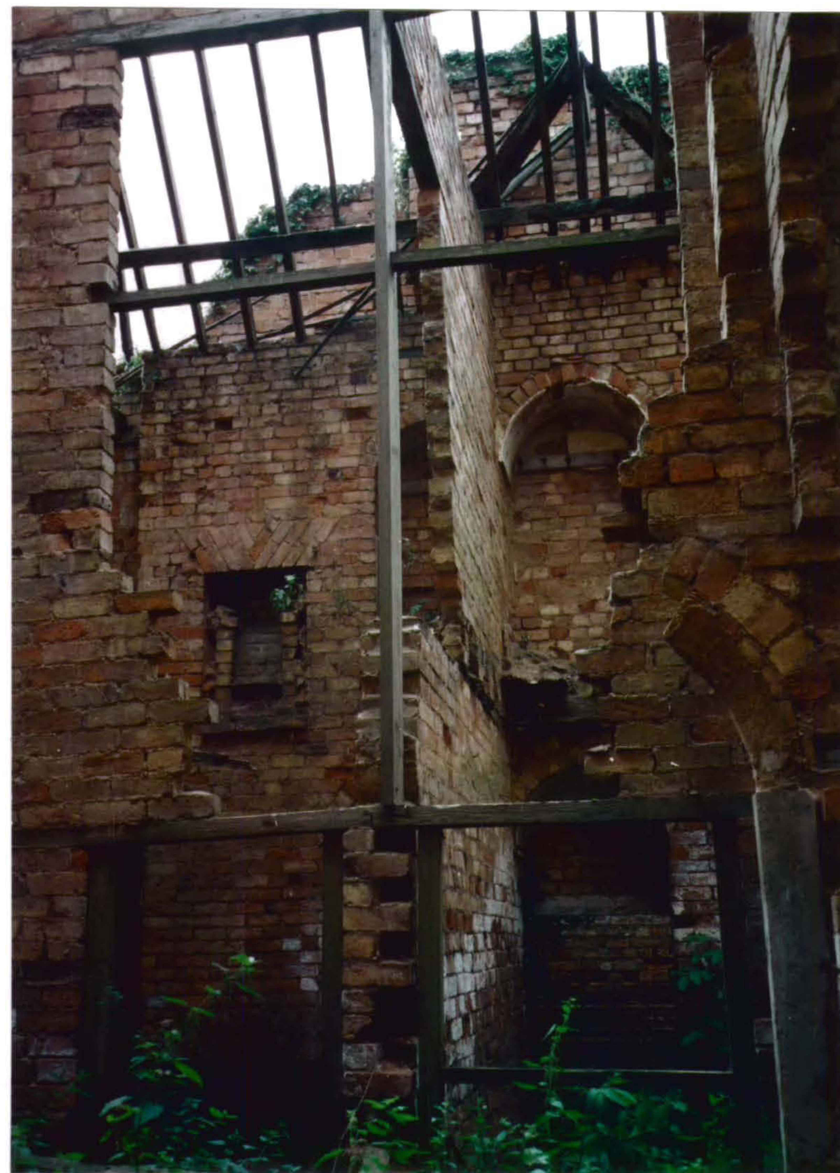
Plate 22 Interior view of the residential area of the South Range – left of the entrance. Revealing substantial sections of single brick walls at first floor. The brickwork of the alcoves and fireplaces are characteristic of those found throughout the house.
