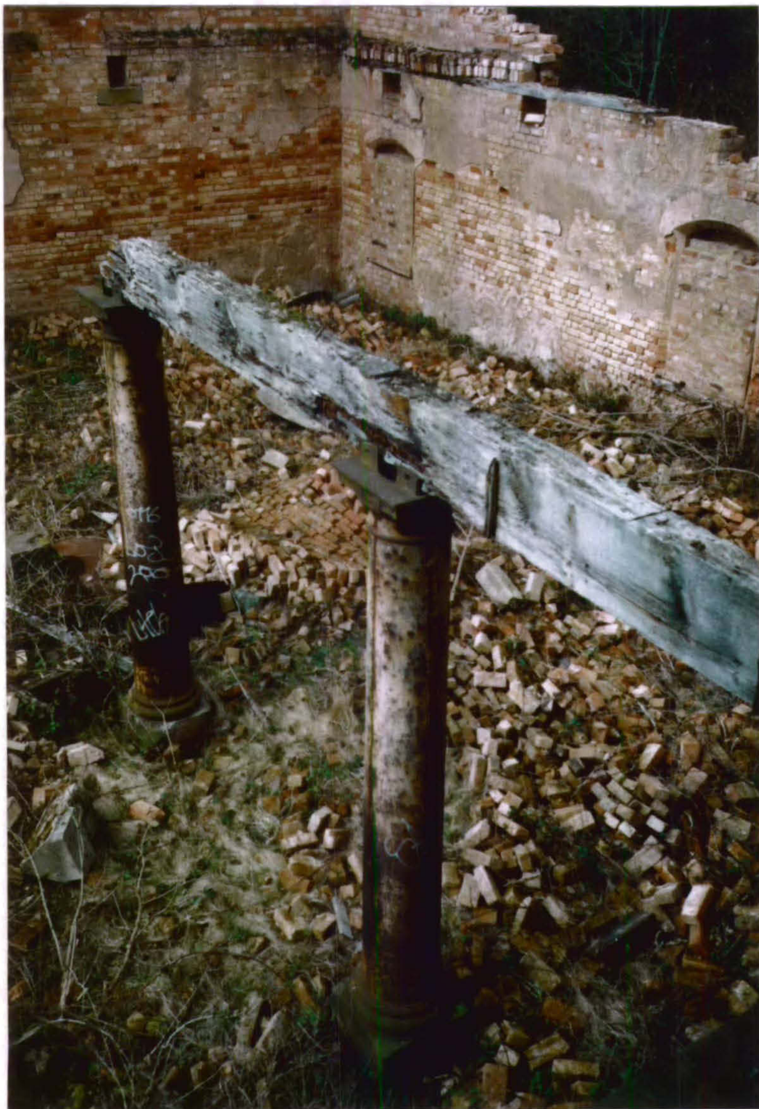
Plate 13 Detail showing two cast-iron columns and floor beam surviving in situ. North Range - Carriage House.
