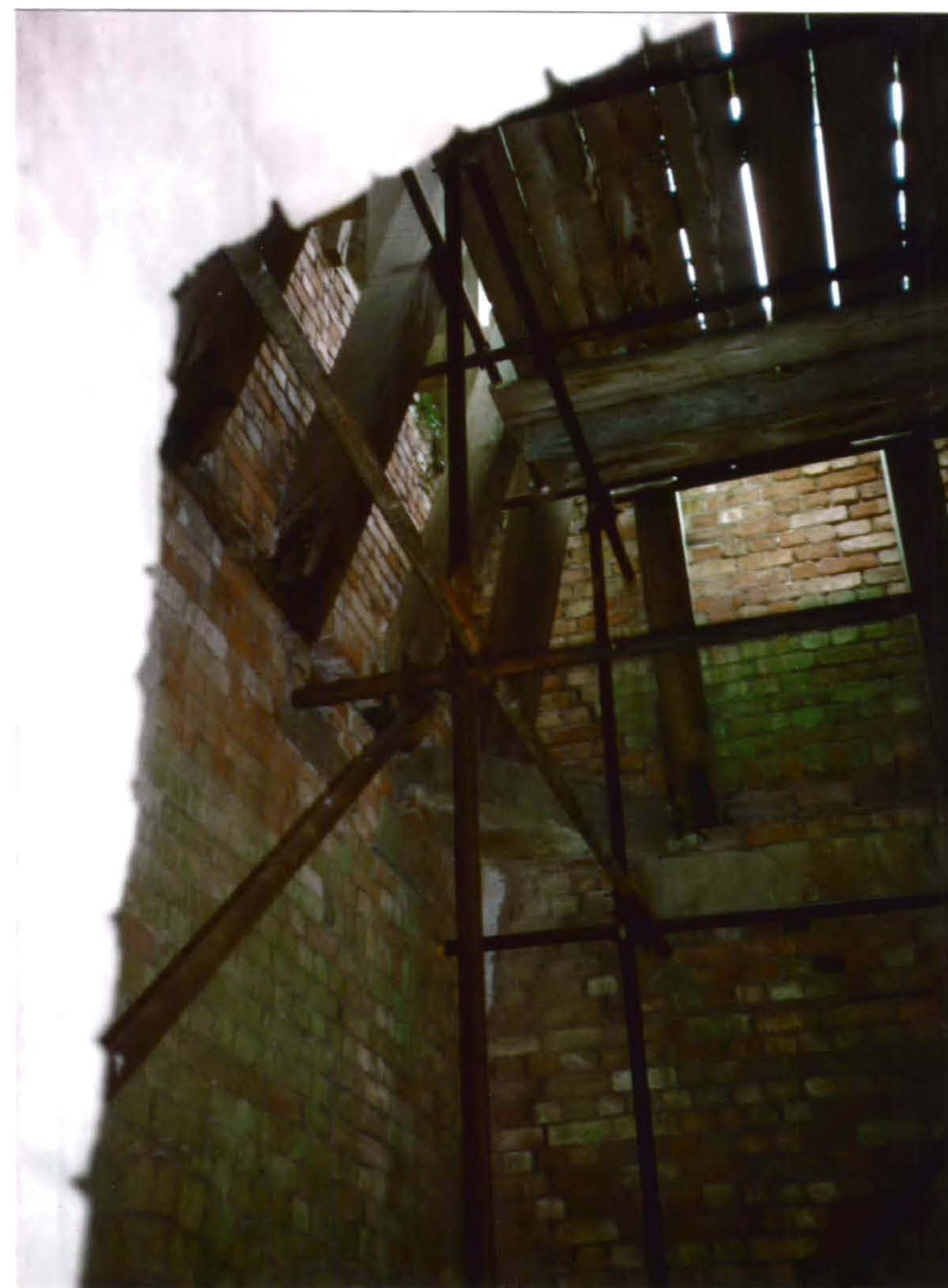
Plate 20 Detail view of part of the framing to support the clock mechanism in the Clock Tower. Also shows the scaffolding installed c.1992 to reduce the load on the weakened timber framing.
