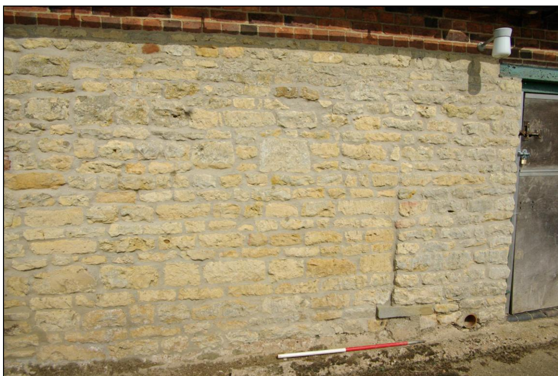
Figure 8. Step or repair in south wall of Barn A (eastern section).
