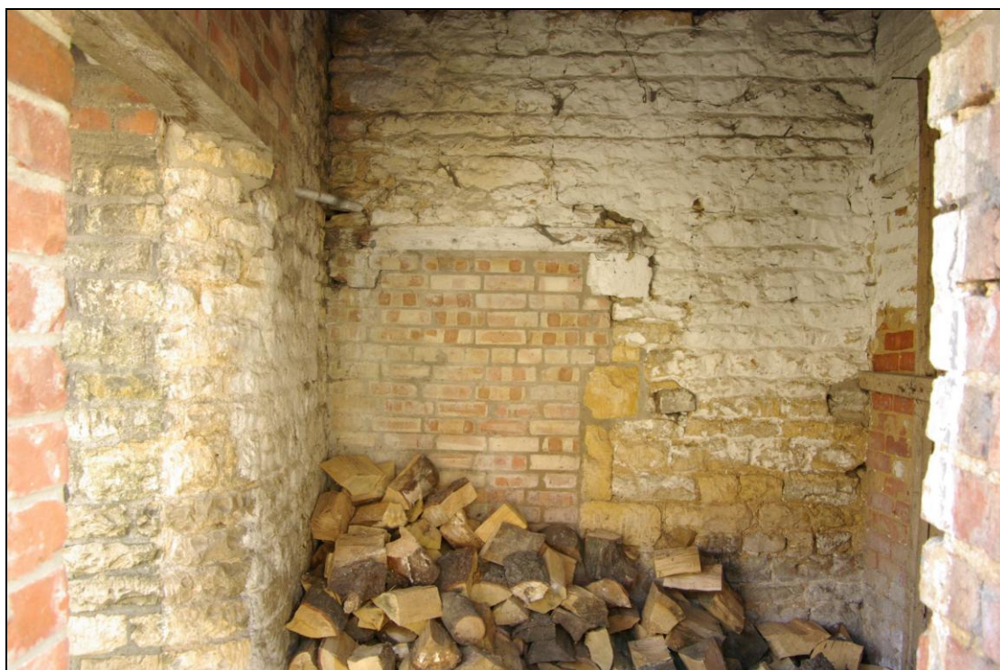
Figure 14. Blocked doorway on north wall of Barn A (western section) viewed through rear outbuilding doorway.
