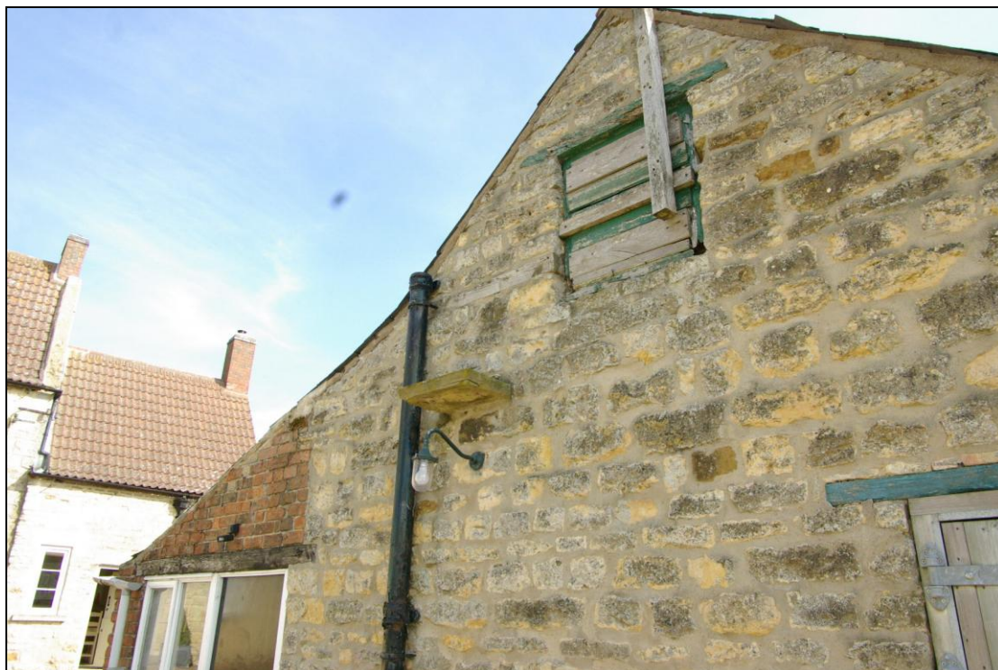
Figure 13. Western gable end of Barn A showing limestone plinth and rear outbuildings.
