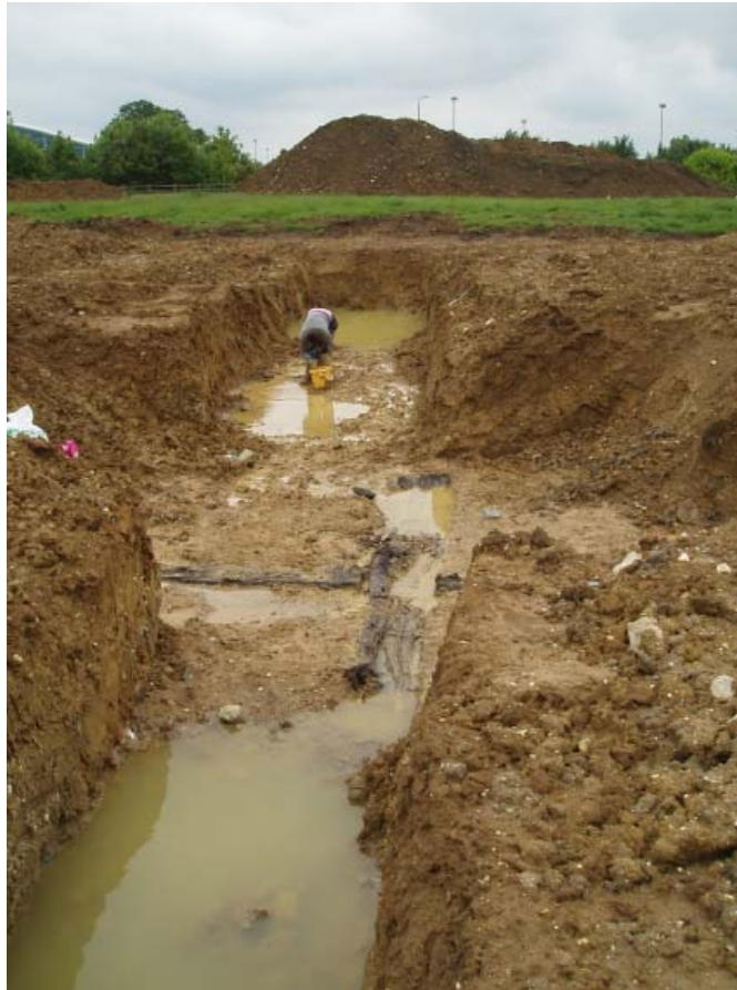
Plate 1 The excavated trench through the windmill mound looking east with the cross-trees in the middle ground
