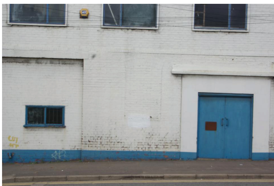
Figure 12 Plot 30 (ii) Blocked Window Detail.
