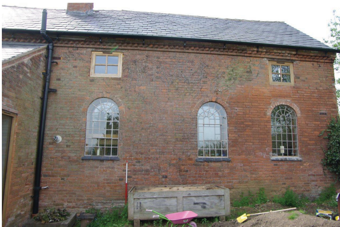
Figure 11 North elevation detail after insertion of new windows New windows are first floor on left and ground floor on left Looking south. 1m scale
