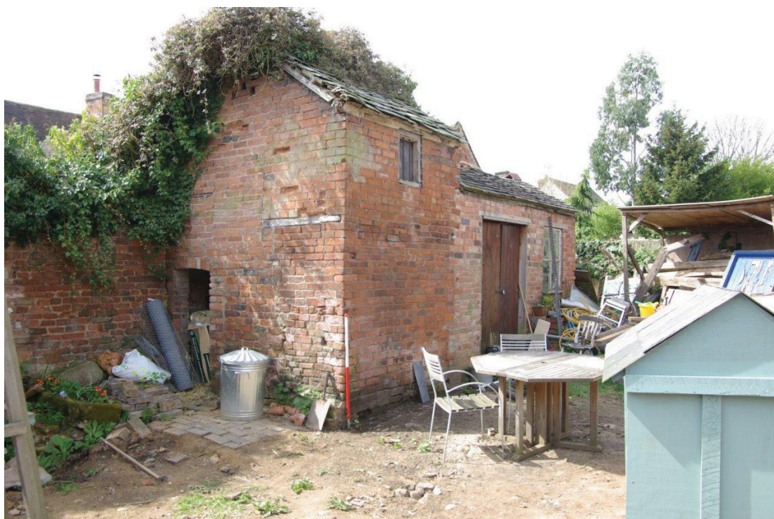
Figure 8 Outhouses to the south of the main building Looking south west. 1m scale
