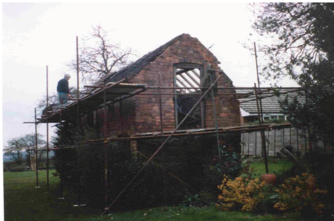
Plate 2: The demolished outbuilding that had existed in centre of site, looking north. Picture provided by J. Rowland,
