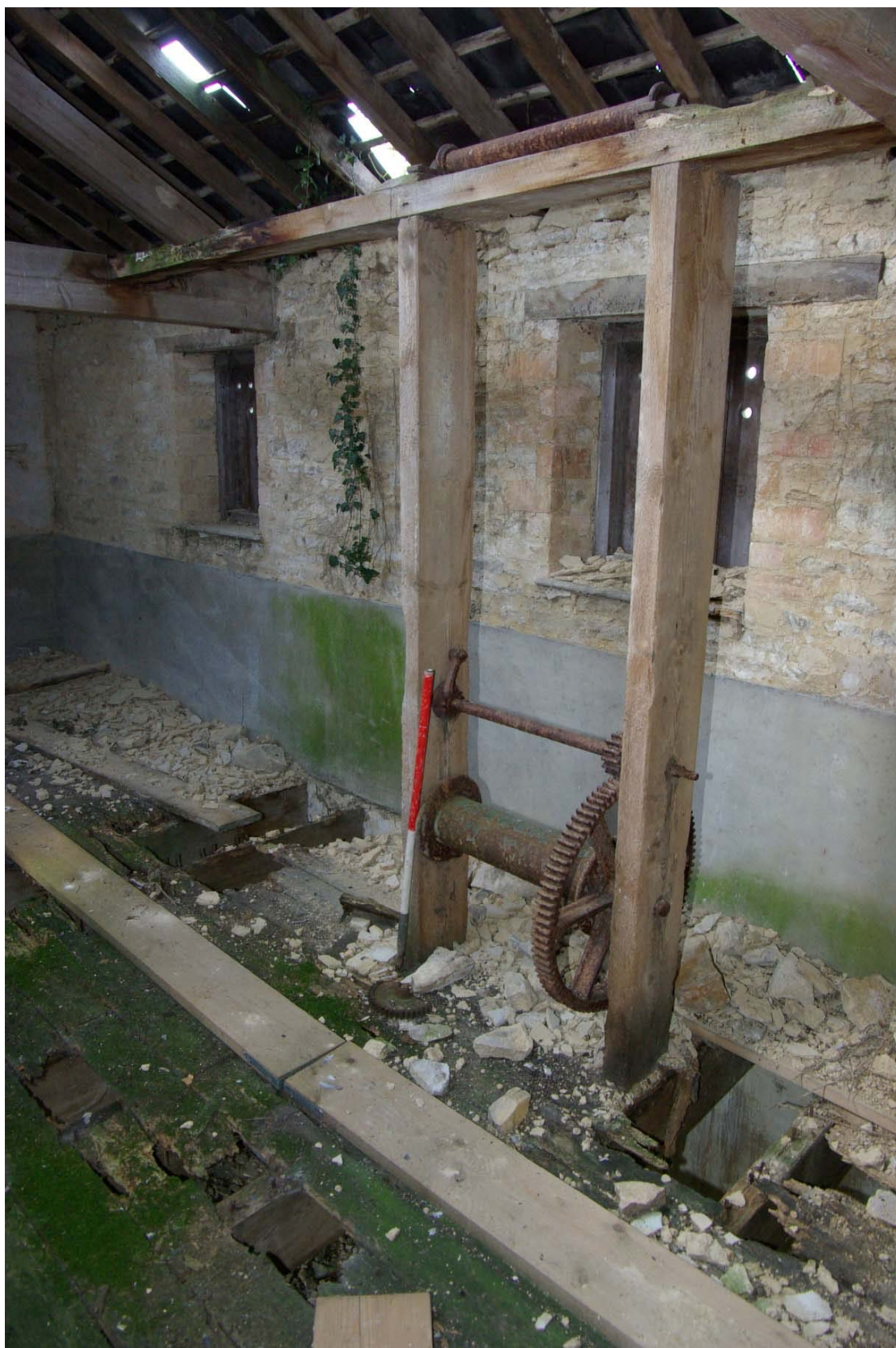
Figure 41 Room 13 winding gear Looking north west. 1m scale
