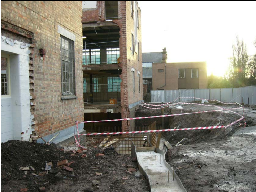
Plate 3. Modified façade of Boston House looking east. Piled foundations in front of both buildings.
