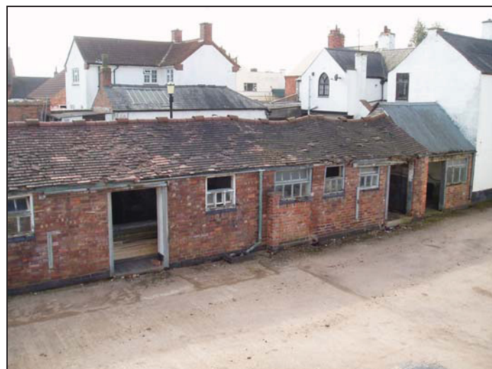
Figure 2: General view of the outbuildings (looking south west). Outbuilding A (easternmost building) and part of B are in the left-hand picture, B, C and D (westernmost building) are in the right.
