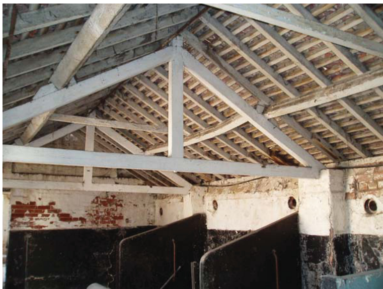
Figure 3: A roof truss in Building B. Note how the king post extends above the apex of the principal rafters allowing the purlins to rest on top of the rafters without the need for jointing. The purlins are prevented from slipping down with a wedge of wood nailed to the rafter.
