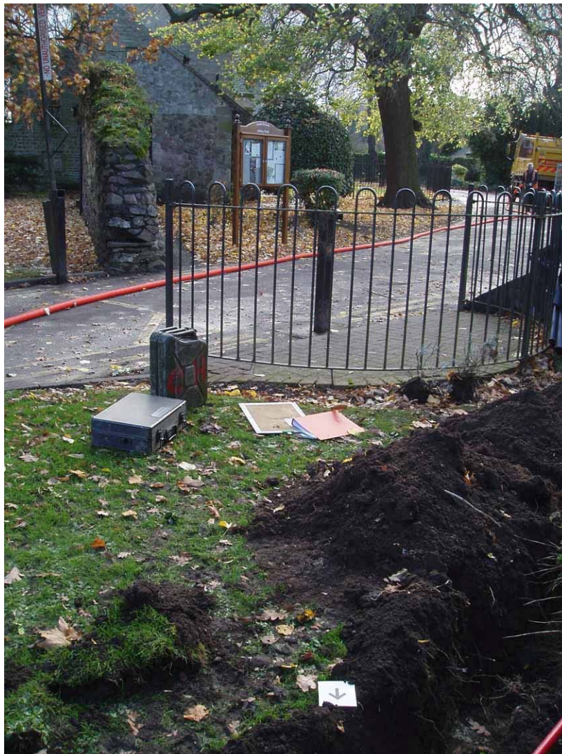
Figure 6 Trench and surviving halt-way wall Excavated foundation in foreground below north arrow
