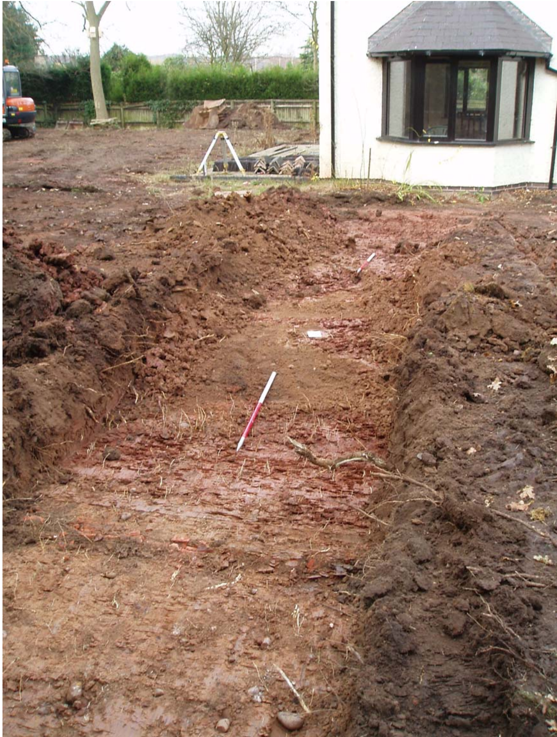
Figure 5: Trial trench viewed from the east in area of plot 1. The existing building in the background forms Plot 2.
