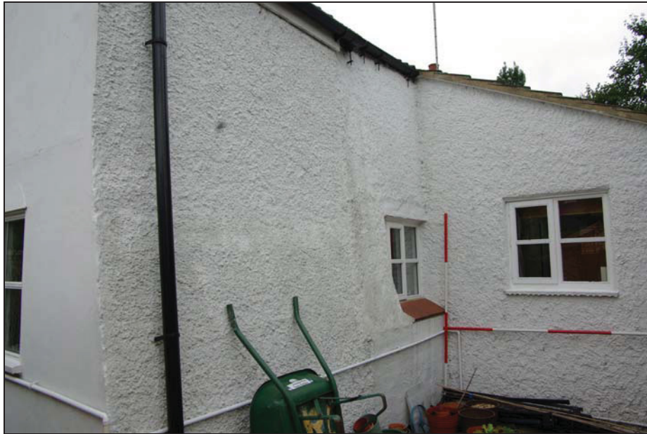
Plate 8: The north-east corner of the property showing the original cottage (centre) and extensions to the east (two-storey, left of picture) and north (single storey, right) elevations.
