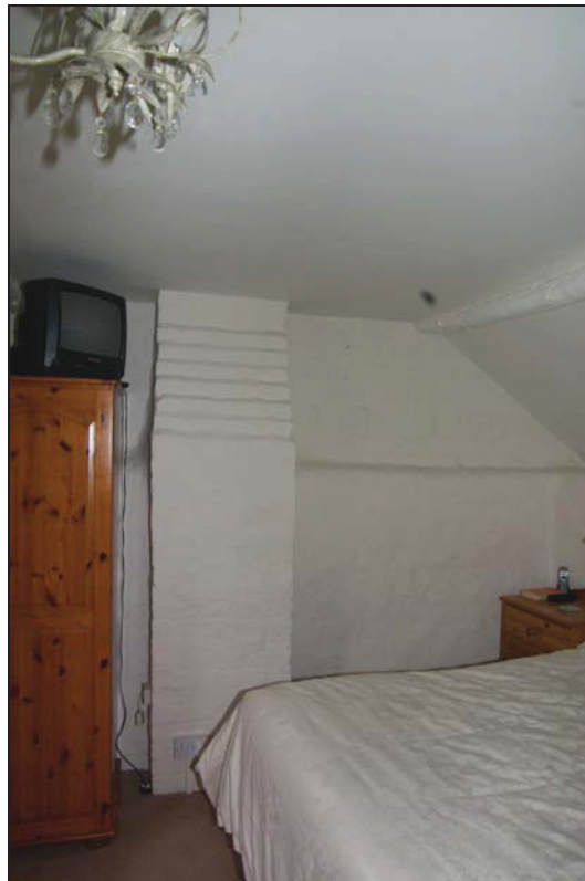
Plate 6: Interior wall of the western elevation (bedroom 1), showing the cob wall joining the upper brick gable end of the house, and the brick chimney stack. Note the roof purlins are timbers kept 'in the round'.
