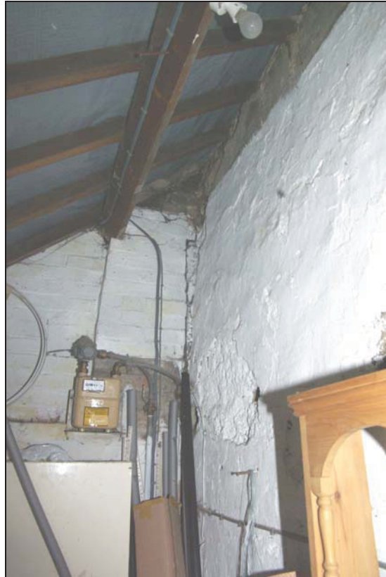
Plate 7: The interior of the outhouse showing the rendered end of the cob wall (the exterior western elevation of the original cottage).
