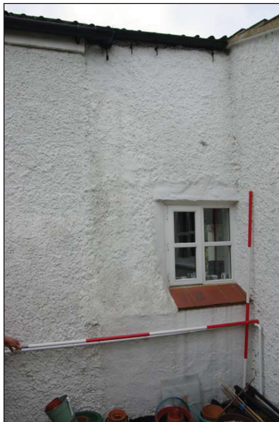
Plate 9: The original north wall of the cottage with replaced window joining the two-storey east elevation.
