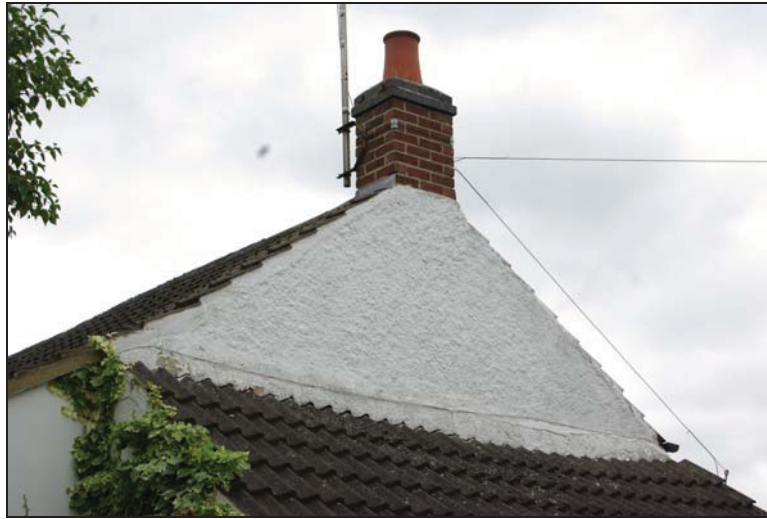
Plate 5: The top of the cob wall on the western elevation joining the upper brick segment gable wall, just above the roofline of the outhouse. The red brick chimney stack with modern pot were presumably added when the cottage was re-roofed with pan tiles.
