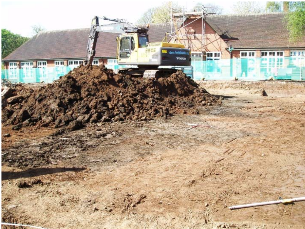
Plate 1 Machine stripping over the pond feature located on the west side of the development area (cut 10).
