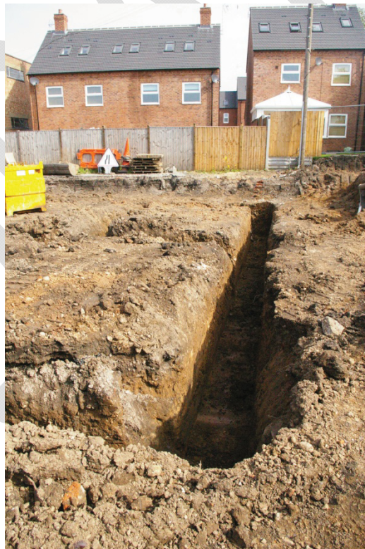
Figure 5: Foundation trench for new dwelling located at the rear 22-24 Loughborough Road Shepshed
