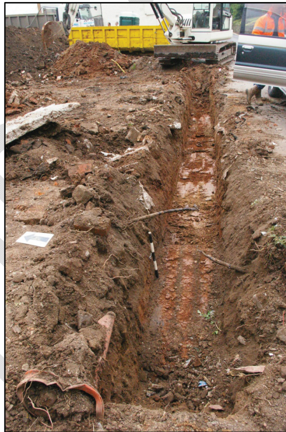
Figure 3: Foundation trench for new dwelling located on the Vine House plot Loughborough Road Shepshed
