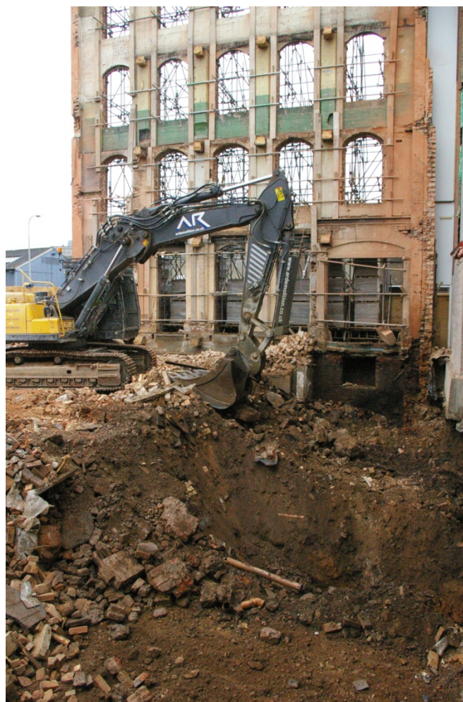
Plate 1 Machine removing demolition material from the basement with the retained 24 Peacock Lane façade in the back ground.
