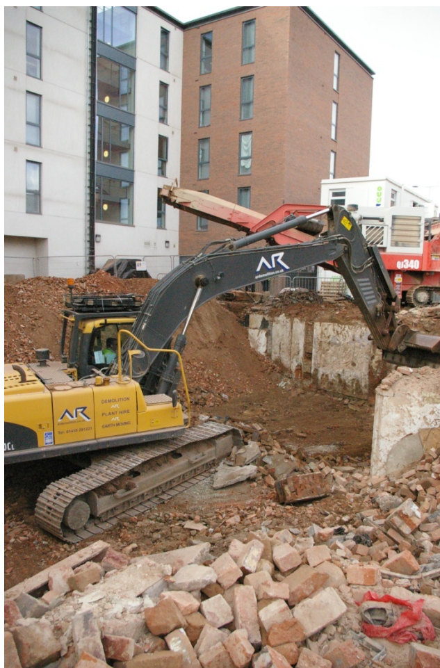
Plate 2 Machine removing basement floor slab located on the north side of the development.
