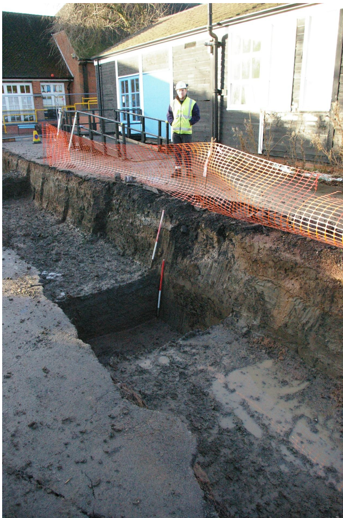
Plate 3 Excavated test slot at centre of Trench 1 into a potential pond or moat.
