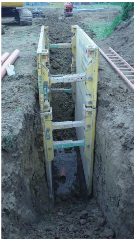
Figure 7: View north of north - south drain slit trench with steel shuttering and drain in base.
