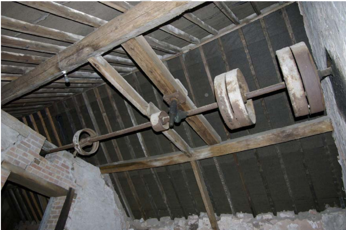
Figure 12 Line shaft within A3 (069-070).
