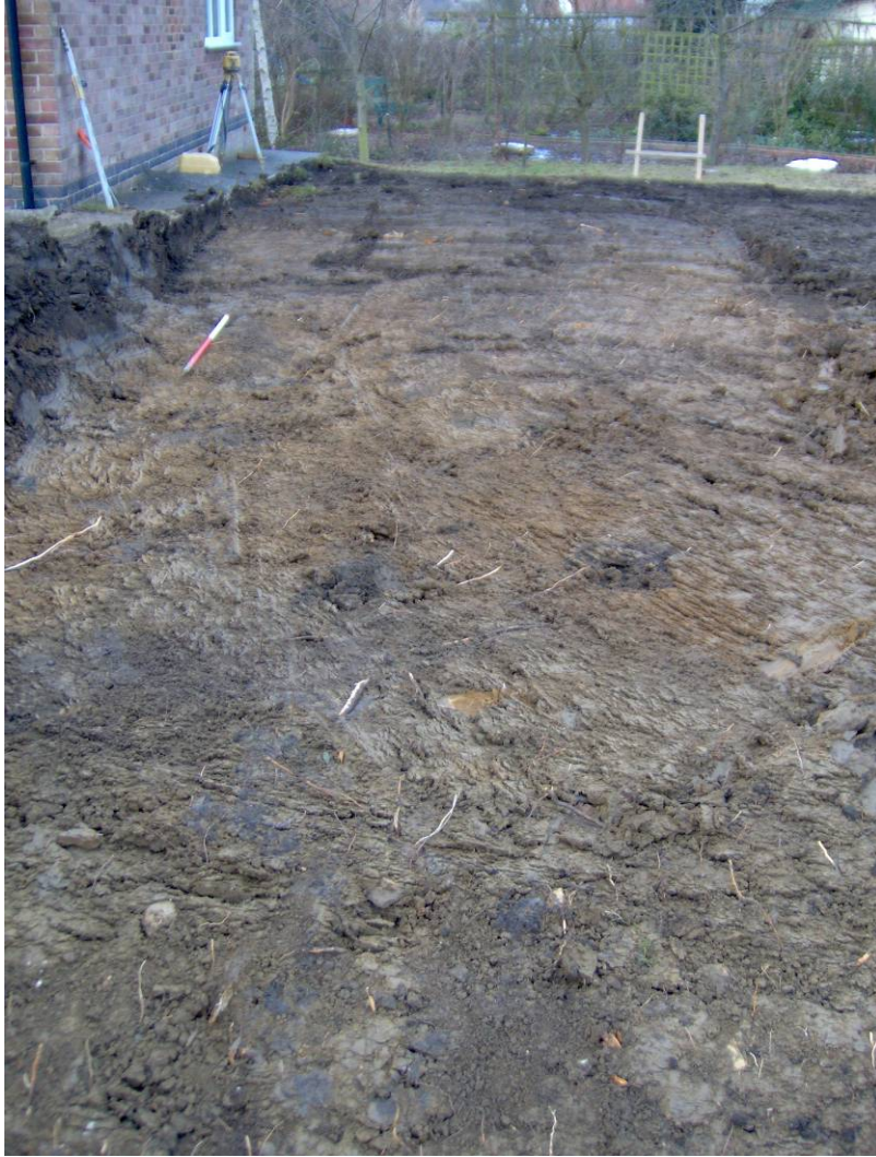
Plate 3: The southern part of the site, to the north of the bungalow, stripped of topsoil, looking west north-west
