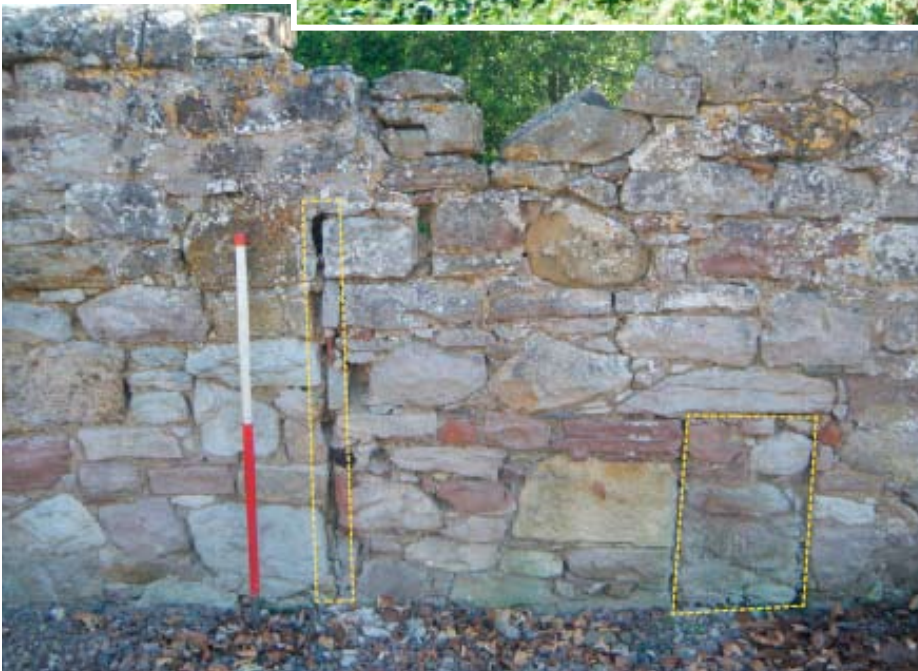
Illus 9 Detail of F2 (right) and F3 (left) on the SW facing elevation
