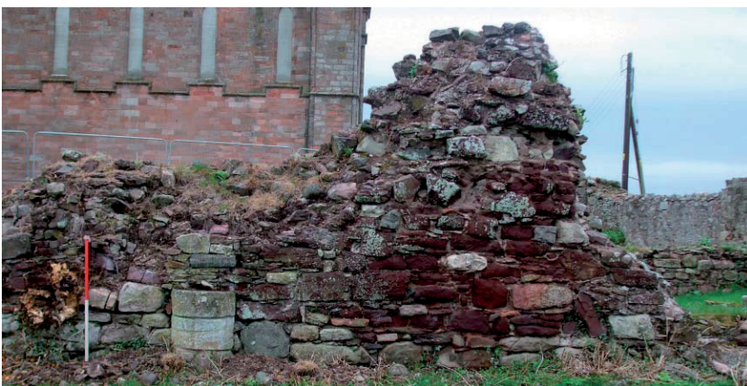
◀ Illus 7 Refectory wall with tree stump within
