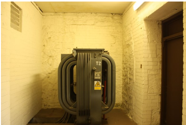
Illus 20: Eastern guardhouse, Transformer 2 in Room 2
