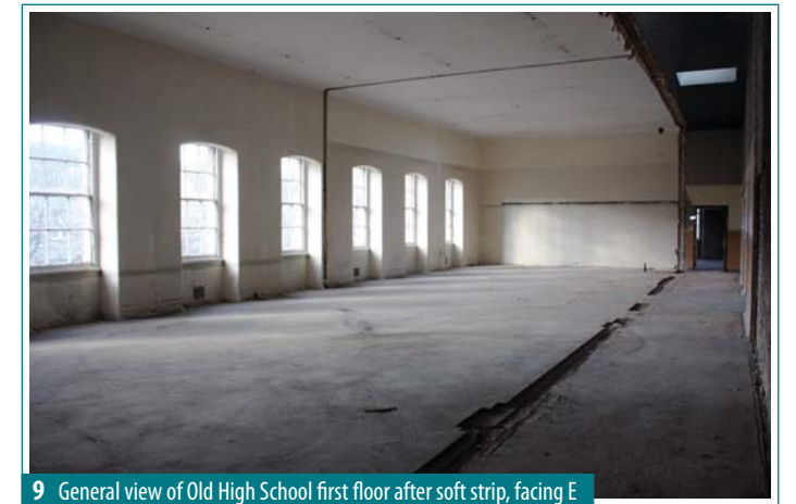
9 General view of Old High School first floor after soft strip, facing E
