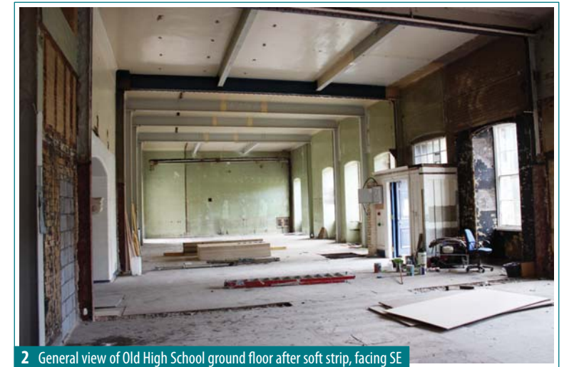
2 General view of Old High School ground floor after soft strip, facing SE
