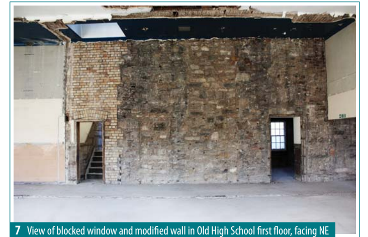
7 View of blocked window and modified wall in Old High School first floor, facing NE
