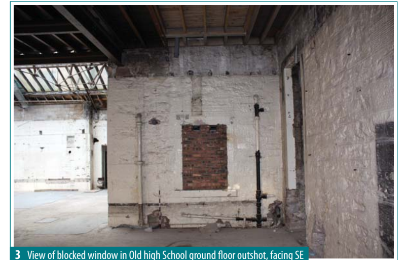
3 View of blocked window in Old high School ground floor outshot, facing SE
