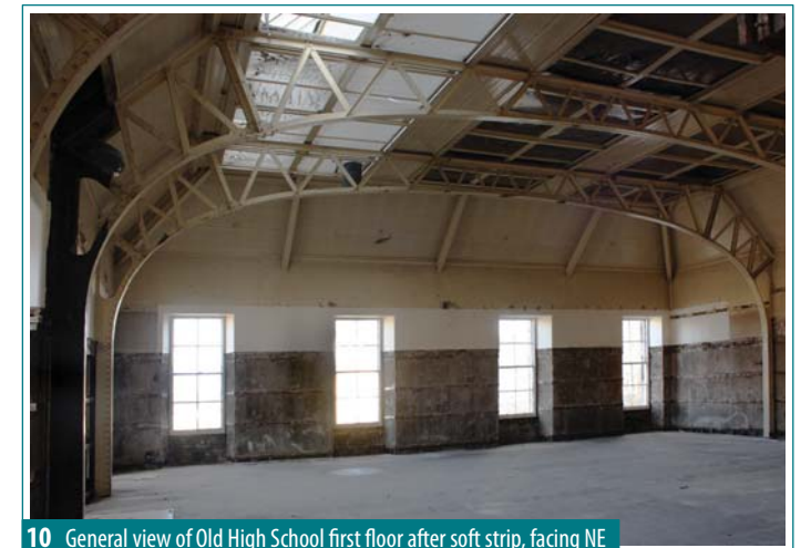
10 General view of Old High School first floor after soft strip, facing NE
