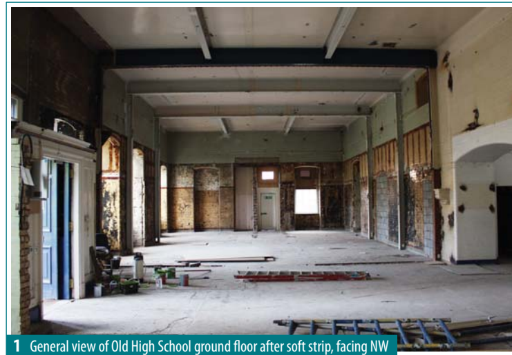
1 General view of Old High School ground floor after soft strip, facing NW
